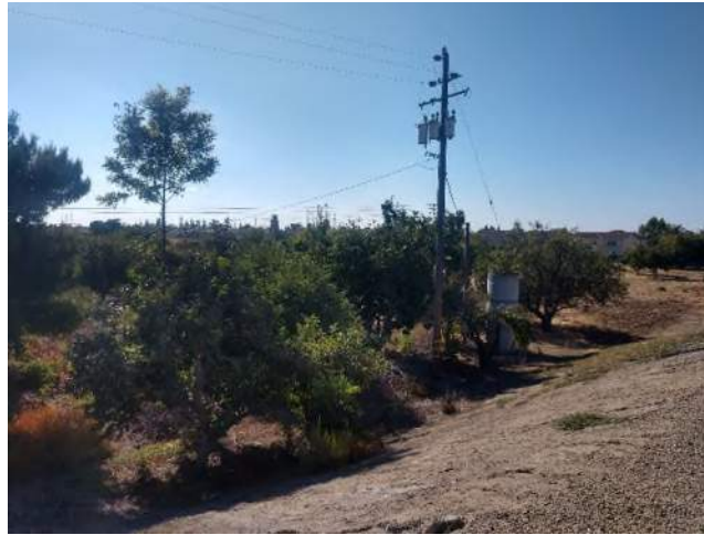
Figure 17 – View of transformers adjacent north near levy.
