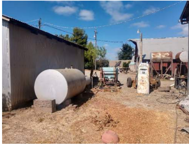
Figure 5 – View of AST and gas dispenser.
