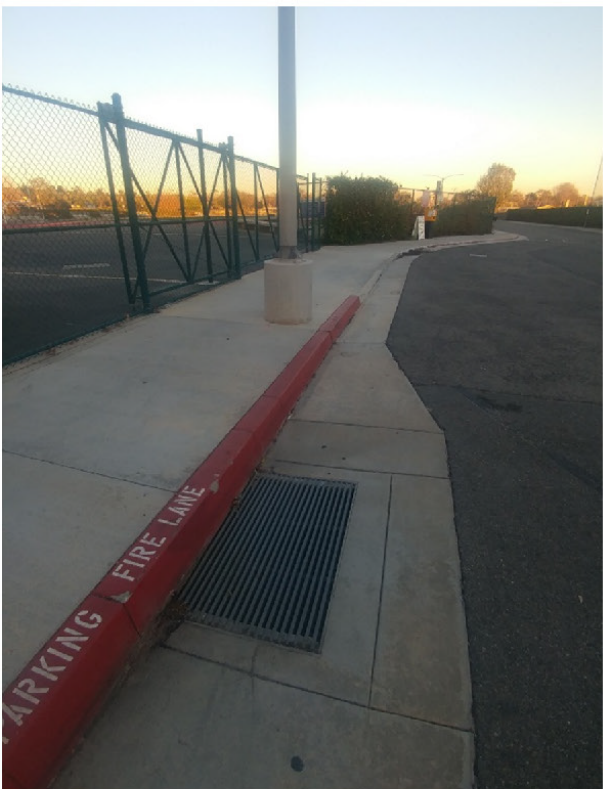
Catch Basin South of the site to be used for overflow conditions
