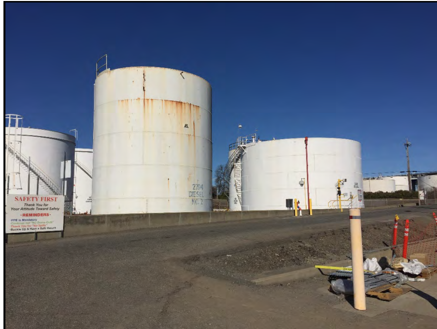
Photograph 2. Overview of tanks and driveway at 76 Broadway. Image taken February 2018; view northwest.
