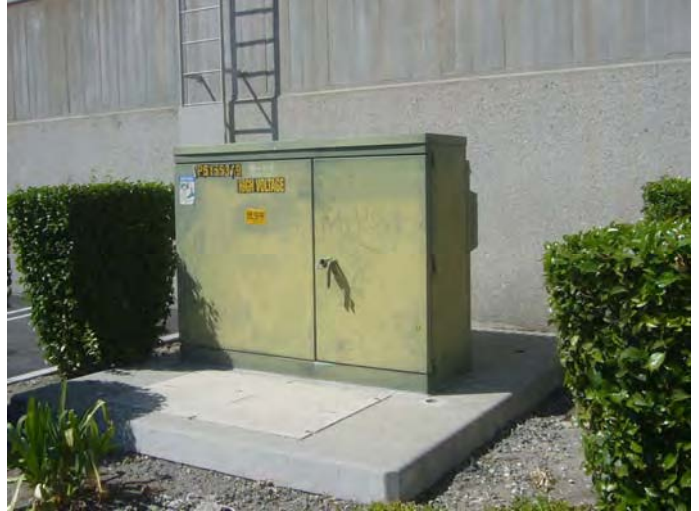
6) View of a typical electrical transformer.
