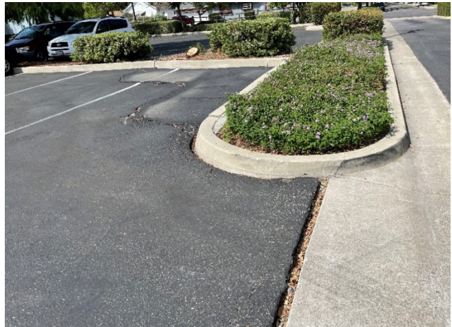
Notable gaps were observed between sections of the asphalt pavement and stormwater drainage route.
