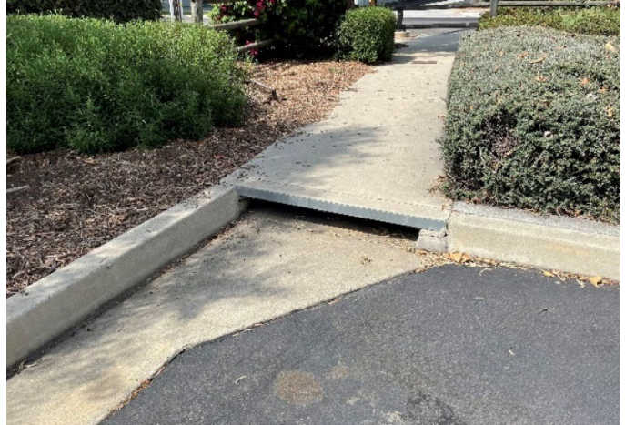
Storm drain system curb-opening inlet at the southwest corner of the Subject Property.
