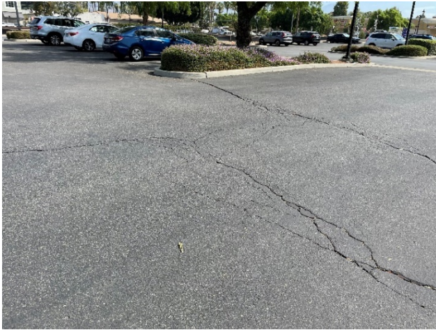
Minor asphalt cracking was observed throughout the outdoor parking facility.
