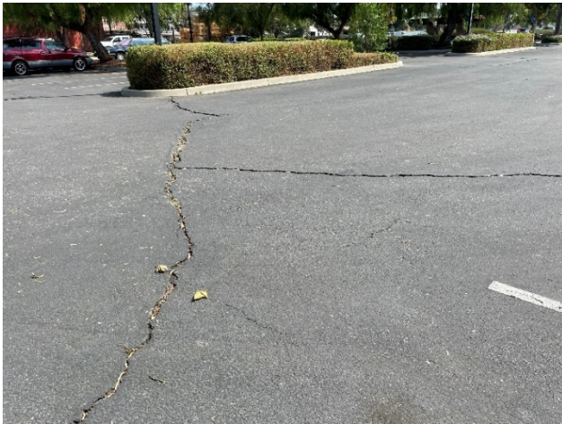
Wider and deeper cracks have a higher potential to enable leaching into the subsurface soil.
