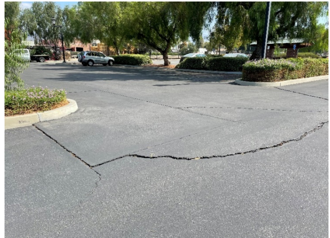
Significant cracking was noted at the southwest corner of the Subject Property.
