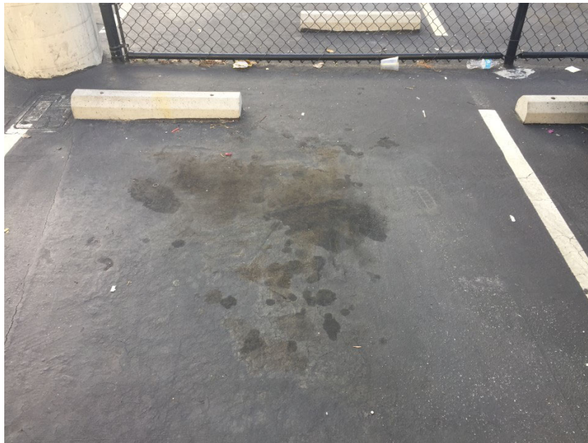
Photo 2. View of minor staining typical of asphalt-paved parking areas. Photograph taken January 25, 2017.
