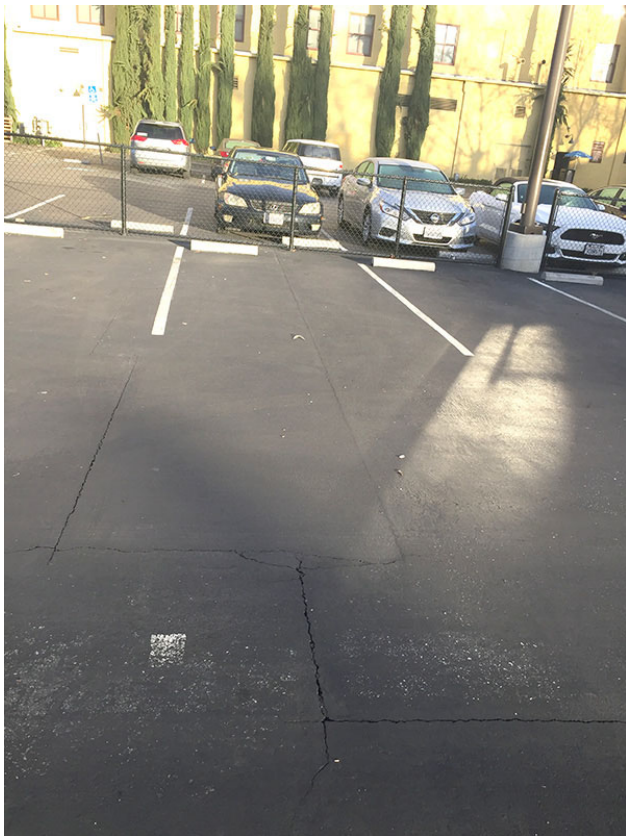
Photo 1. View of typical patched and/or cracked asphalt. Photograph taken January 25, 2017.
