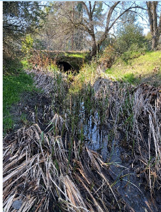
Photograph 5: Southern end of project boundary with Oak Park Boulevard culvert in view, looking south
