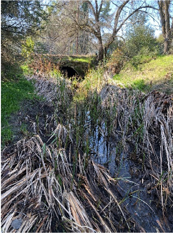
Photograph 5: Site 1, southern end of project boundary with Oak Park Boulevard culvert in view, looking south.
