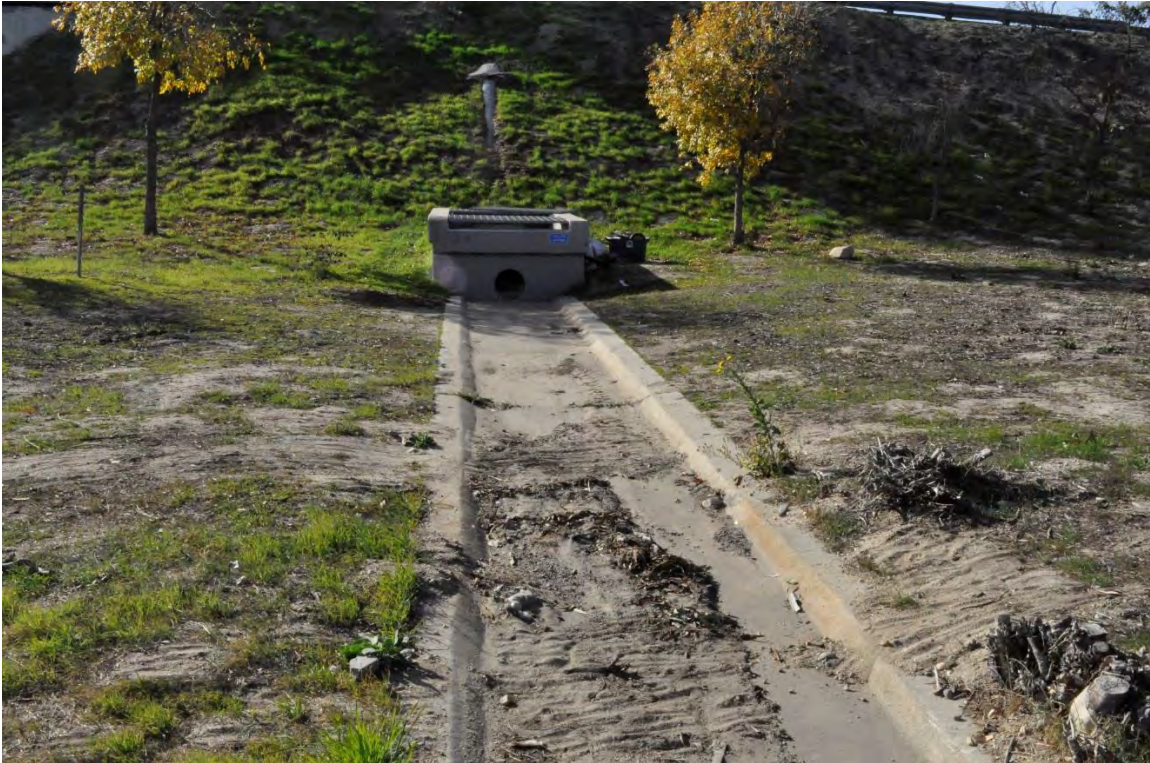
Culvert Perpendicular to Tujunga Wash Central Branch within undeveloped landscaped areas of cloverfield interchange for State Route 170 along Victory Blvd – DSC0134
