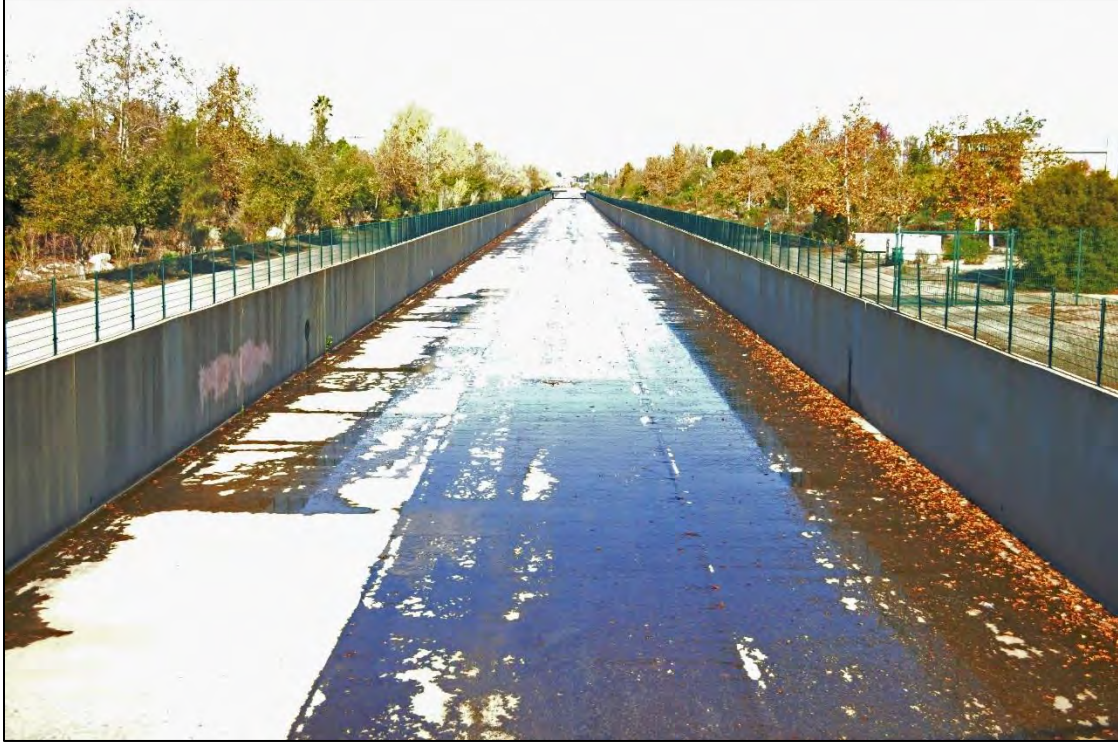
Tujunga Wash Flood Control Channel North of Victory Blvd and west of Coldwater Canyon Ave – DSC0068
