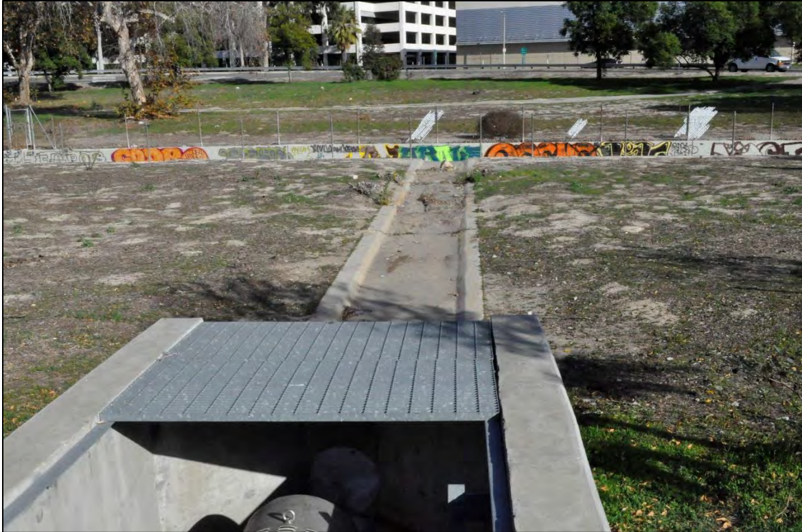
Culvert Perpendicular to Tujunga Wash Central Branch within undeveloped landscaped areas of cloverfield interchange for State Route 170 along Victory Blvd – DSC0135
