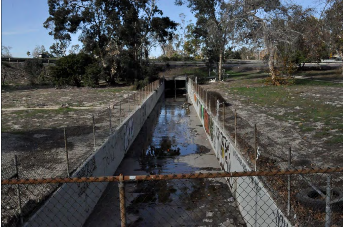
Tujunga Wash Central Branch within undeveloped landscaped areas of cloverfield interchange for State Route 170 along Victory Blvd – DSC0133
