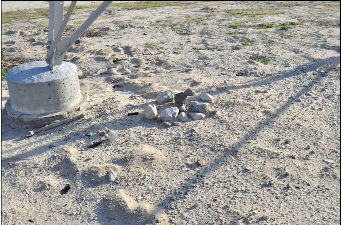
Rocks Under Electrical Towers within Whitnall Highway Utility Corridor South of Victory Blvd–DSC0035
