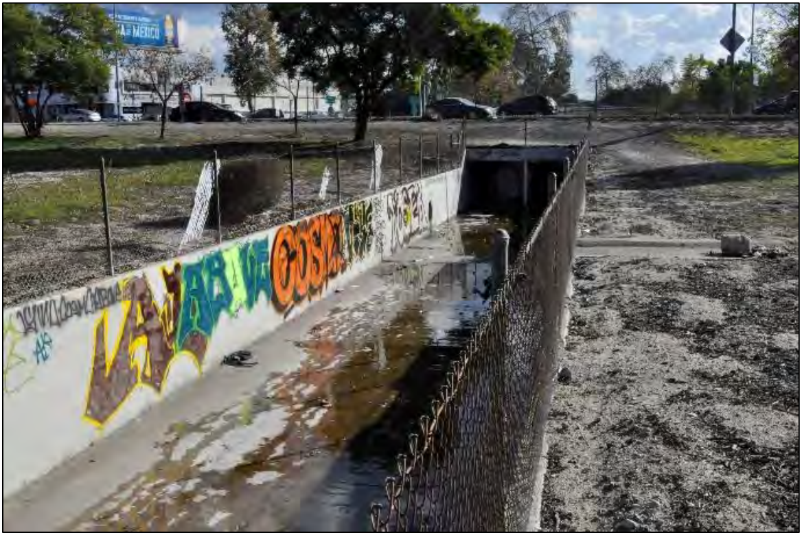
Tujunga Wash Central Branch within undeveloped landscaped areas of cloverfield interchange for State Route 170 along Victory Blvd – DSC0136
