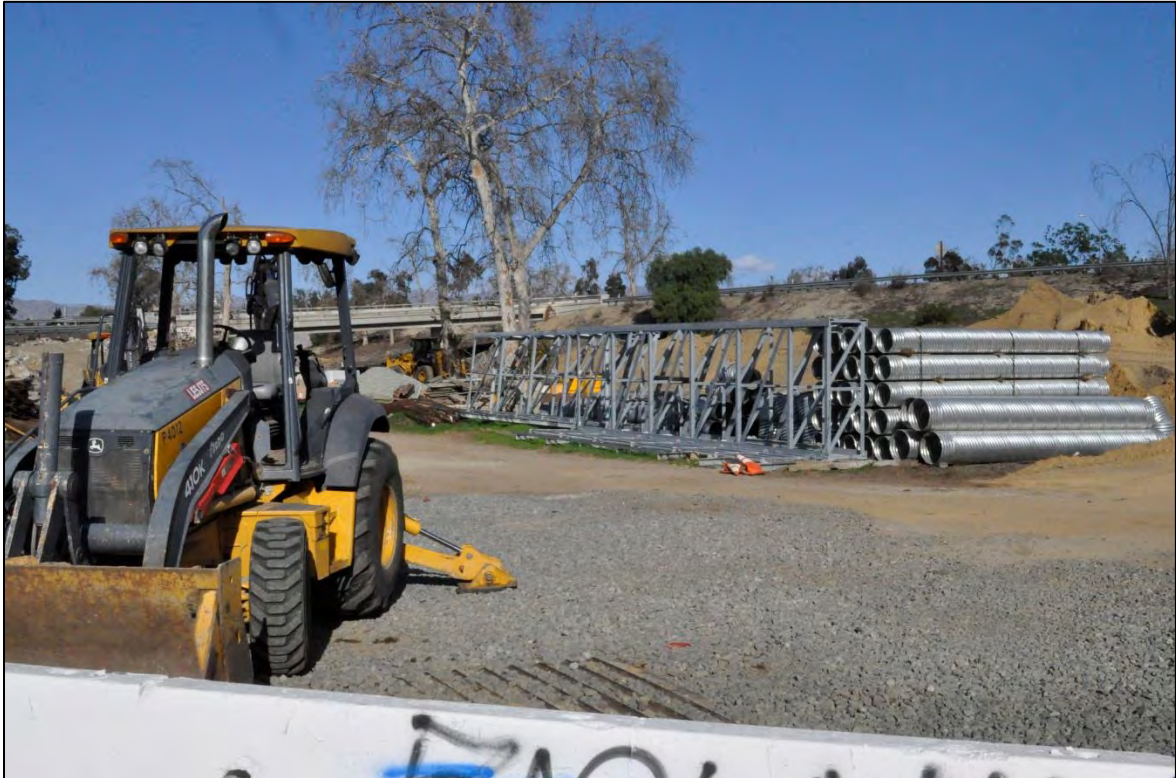
Staging Area within undeveloped areas of cloverfield interchage for State Route 170 along Victory Blvd – DSC0138
