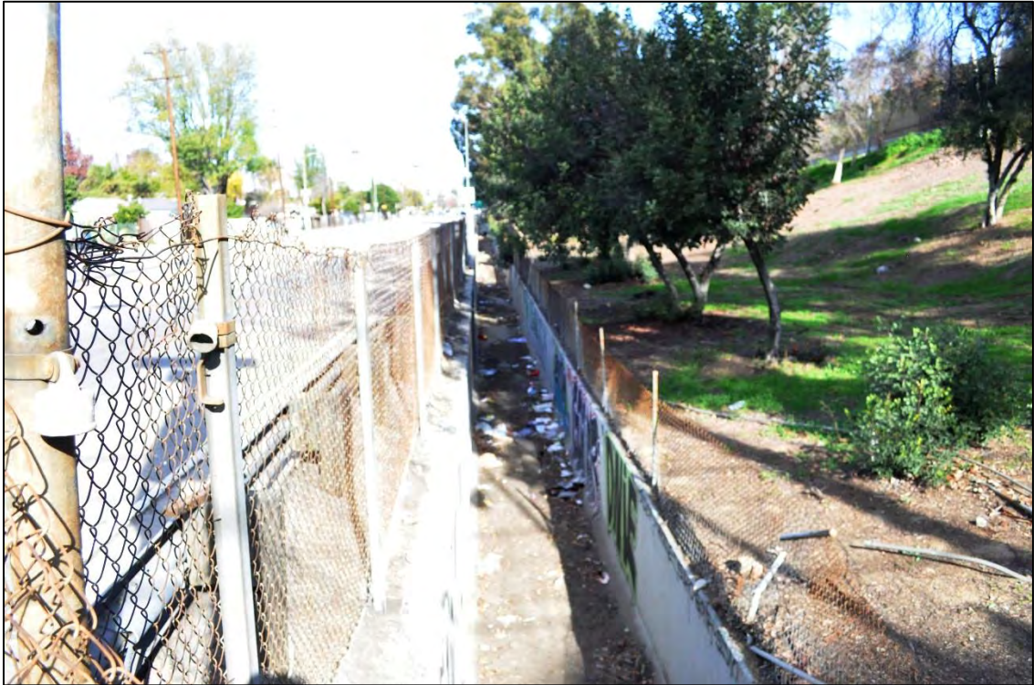
Haskell Creek concrete channel on North East Corner of Victory Blvd and Haskell Ave – DSC0100
