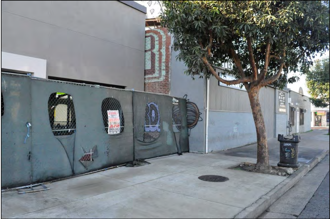
Pump Station Area on South West Corner of Victory Blvd and Lankershim Blvd – DSC0054
