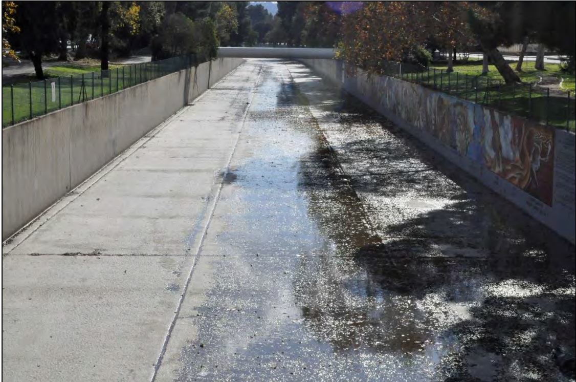
Tujunga Wash Flood Control Channel along Oxnard St. and west of Coldwater Canyon Ave– DSC0119
