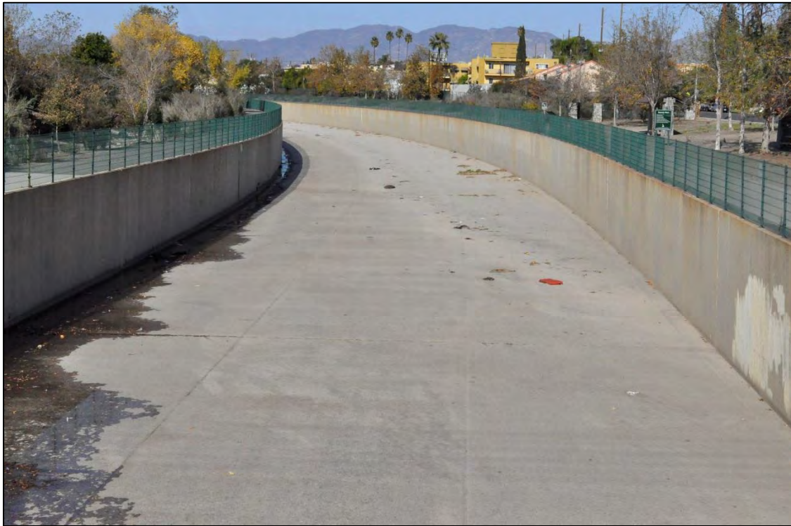
Tujunga Wash Flood Control Channel along Oxnard St. and west of Coldwater Canyon Ave – DSC0117
