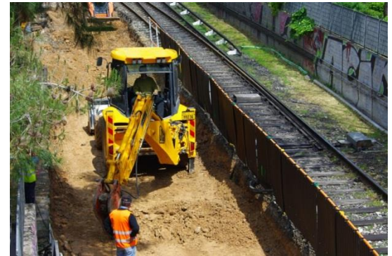
A construction barrier is built at the edge of the site to protect tracks from adjacent work.
