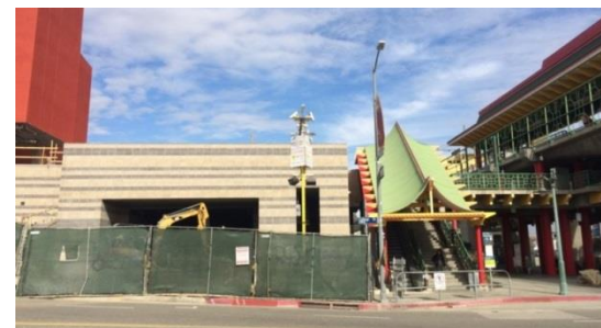
Sidewalk access is blocked for construction project, forcing pedestrians into street or to use less direct paths to the Metro facility.
