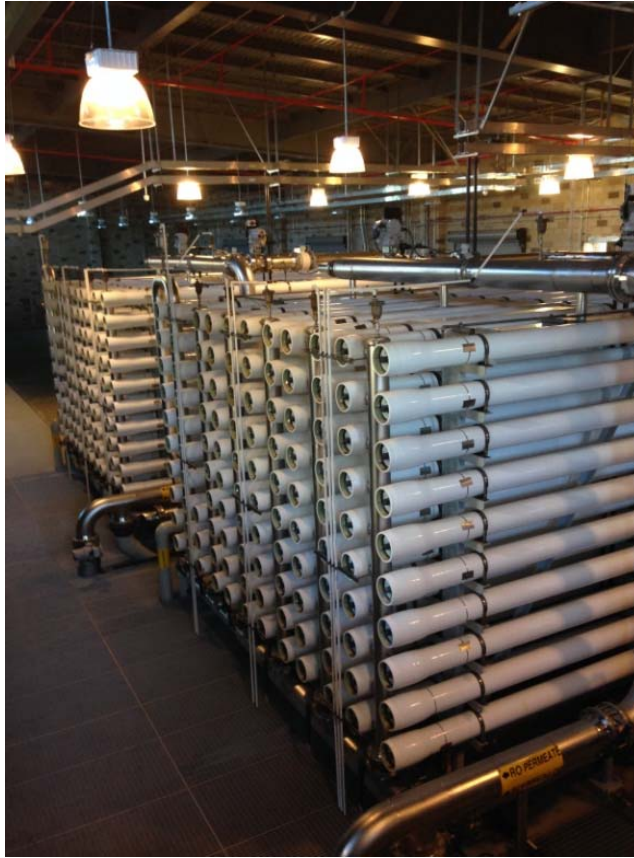
Figure 5 RO Photos at the AWP
