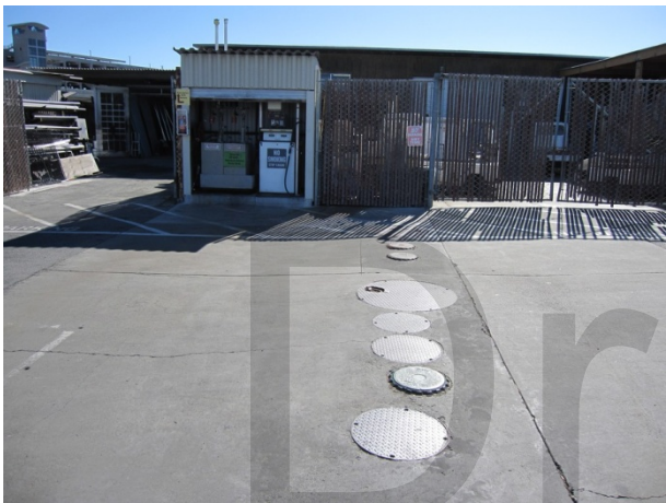
Photograph 11. Dual compartment UST, dispenser and adjacent oil and hydraulic fluid ASTs.
