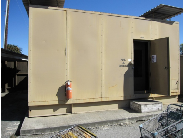
Photograph 15. Emergency generator near water supply well.
