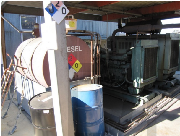
Photograph 5. Two emergency generators and associated diesel AST.
