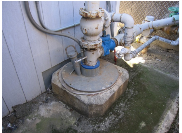
Photograph 14. Water supply well.
