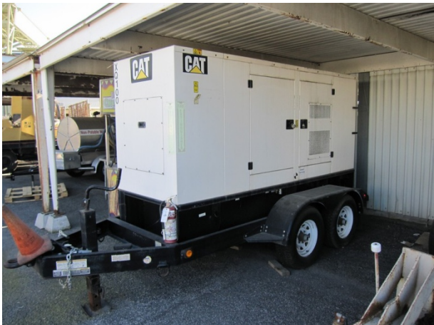
Photograph 7. One of several trailer mounted emergency generators.
