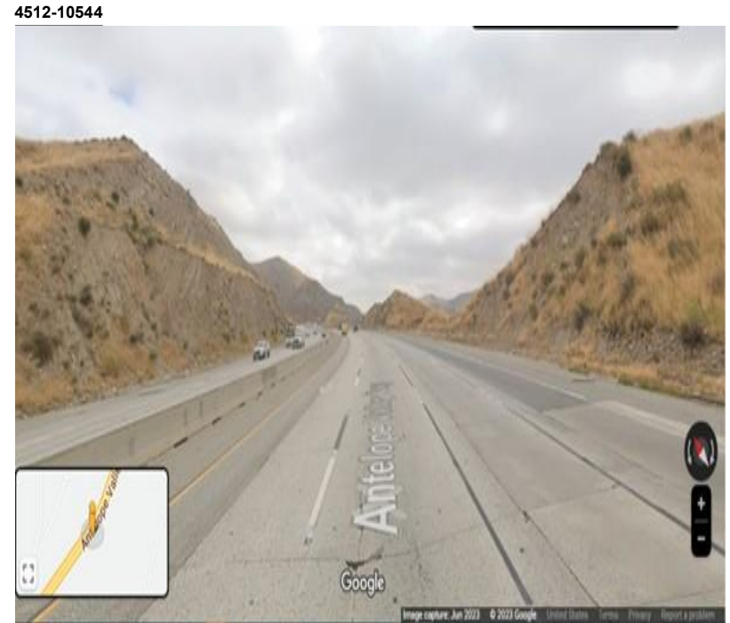
Figure 4. Looking northwest at the steep cut slopes along the SR 14 freeway adjacent to Bee Canyon.
