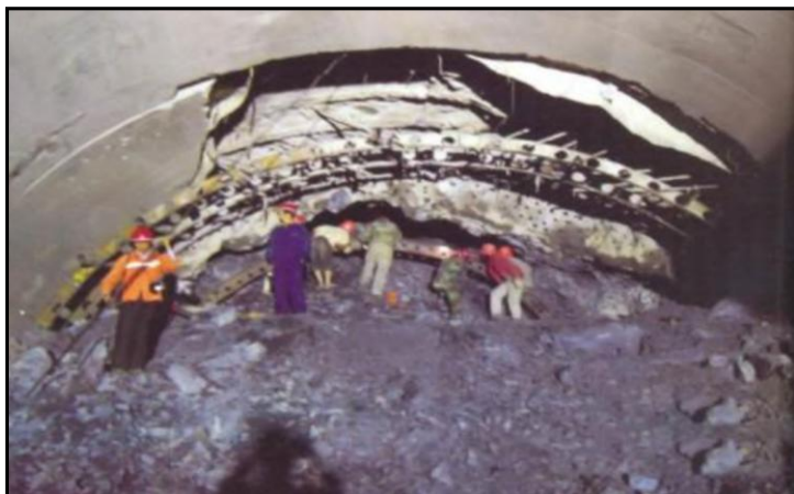
Wenchuan earthquake 2008 tunnel collapse at fault crossing.
