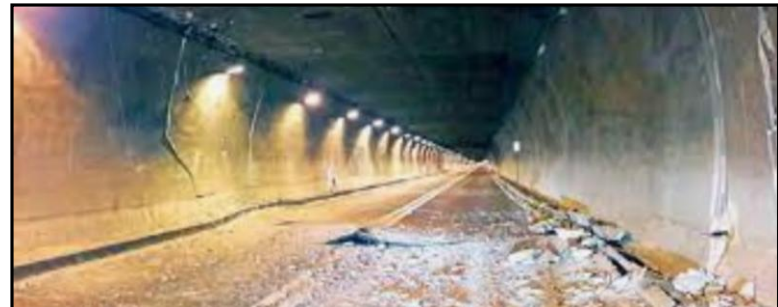
2016 San Benedetto tunnel following the Norcia earthquake in Italy.
