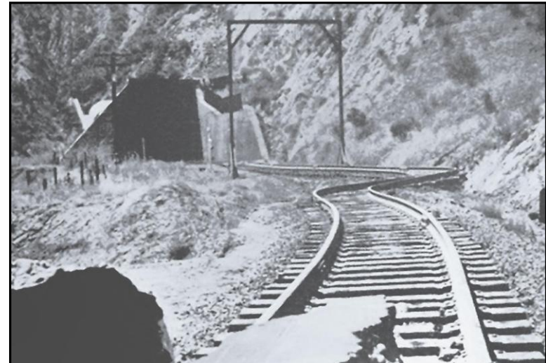
Seismic ground faulting buckled tracks at several locations including inside tunnels in the 1952 earthquake south of Bakersfield.
