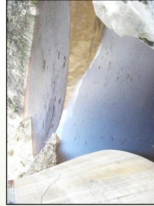
Pacoima Reservoir with sediment and debris after storm following the 2009 Station Fire
