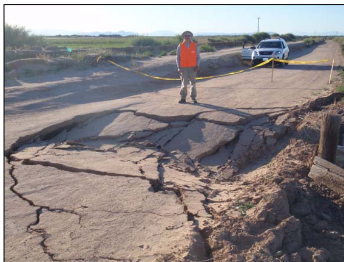
Figure 38. Collapse of the Westside Main Canal's western access road (C05). Undermining of the road surface probably reflects pre-earthquake piping along transverse subgrade structures or other zone of seepage from the canal. No vented liquefied materials were noted in the area. Photo by J. Tinsley, 4/6/10.
