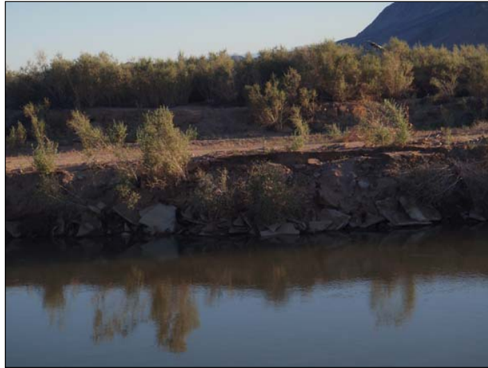
Figure 41. Bank failure probably unrelated to liquefaction in the west bank of Westside Main Canal (C08). This style of failure was observed on both sides of the Westside Main Canal for nearly a kilometer north of State Highway 98. Failures seldom extended more than a meter or two into the levee materials and the bulk of the levees remained undamaged. Photo by J. Tinsley, 4/7/10.
