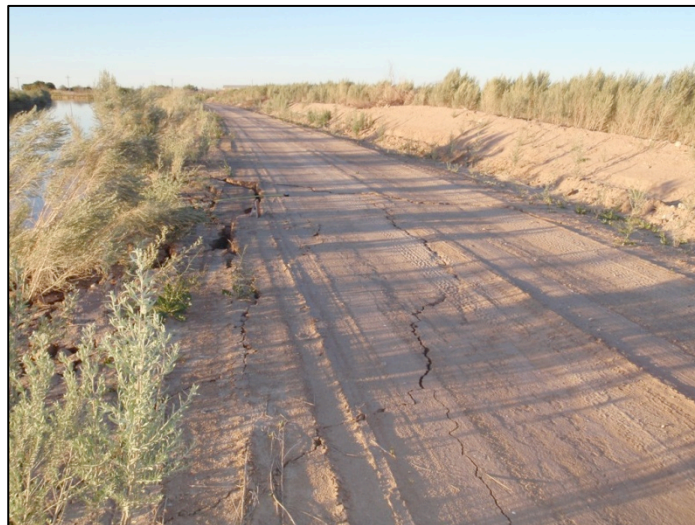
Figure 42. View to north across inferred liquefaction lateral spread in the east bank of the Westside Main Canal (C14). Extensional fractures are open to 95 cm depth and extend across entire width of Westside Main Canal east service road for tens of m. Photo by J. Tinsley, 4/6/10.
