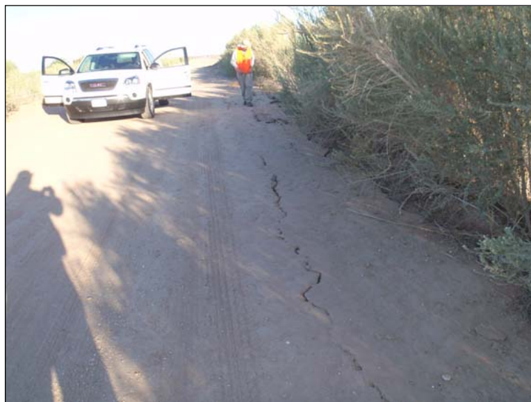
Figure 40. Minor extensional fractures parallel to the channel of the Westside Main Canal (C07). No vented materials were observed in association with this ground failure; the failure is likely a result of strong shaking and not liquefaction. Photo by J. Tinsley, 4/7/10.
