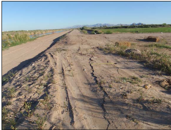
Figure 39. View of extensional fractures at head scarp of lateral spread crossing the embankment in the foreground and including Westside Main Canal's service road to the left (C06). Riparian vegetation is tilted towards the canal owing to lateral spreading. Photo by J. Tinsley, 4/6/10.
