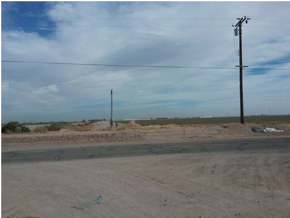
Photo 28: Looking at the drain pump and IID transformer along Drew Road at the concave corner of the subject site.
