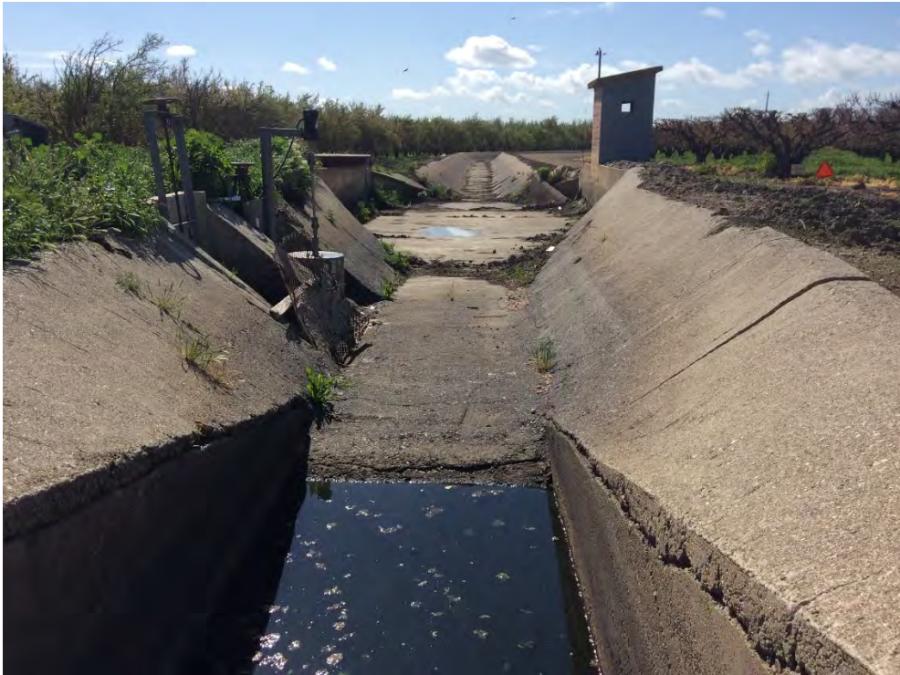
Photograph 4: View of the canal in the northwest portion of the project site facing south.
