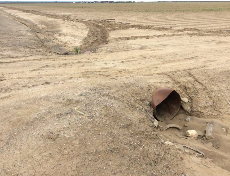
Photograph 4: View of metal drainage pipe in the corner of parcels APN 021-023-025, -024, -020, and -021; facing southwest.
