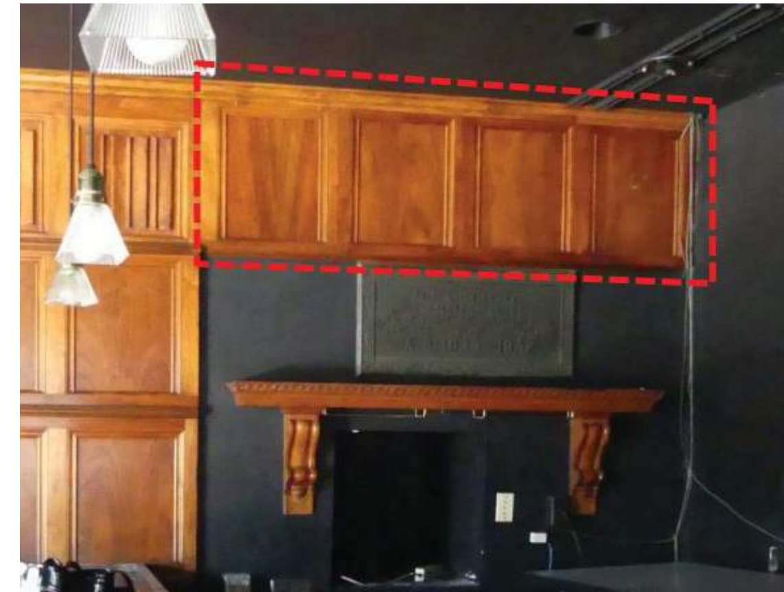
Figure 14. Wood panel and mantle, as installed in Cohiba Club. Source: ESA Report, 2017.
