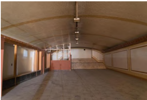
Figure 2: Interior of Jergins Tunnel below Ocean Boulevard, looking north to where the tunnel was closed off, 2016. Source: Michael Wada/Grunion Gazette.
