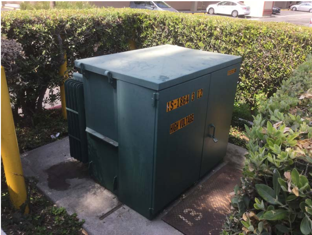
Vaulted transformer near western end of 4325 Glencoe Avenue. 4325 Glencoe Avenue, Los Angeles, California 90292
