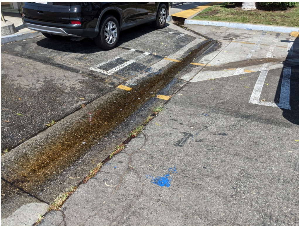
Standing water observed neat Unit C1 at 4325 Glencoe Avenue. 4325 Glencoe Avenue, Los Angeles, California 90292
