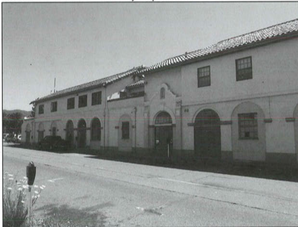
Photograph 4: West side of the building, camera facing northeast. Note second-story addition, parapet flush with addition, and various treatments of ground-level arches.
