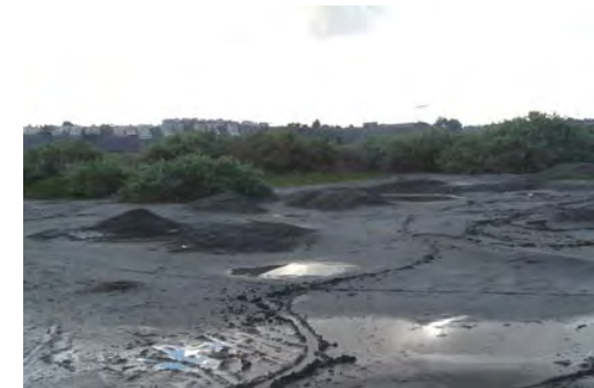
Damage by BMX riders in area A
