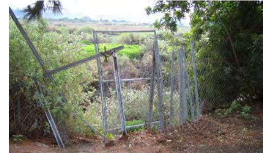
Broken fence at area A
