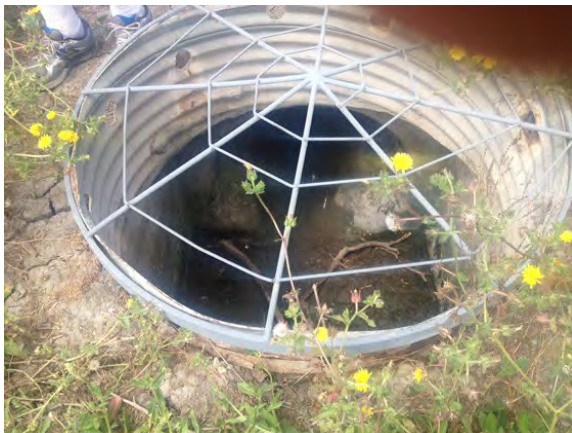
One of the two secret drain openings discovered by photographer Jonathan Coffin
