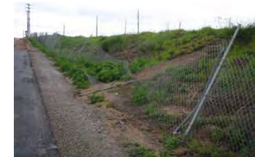
Fallen fence at area C
