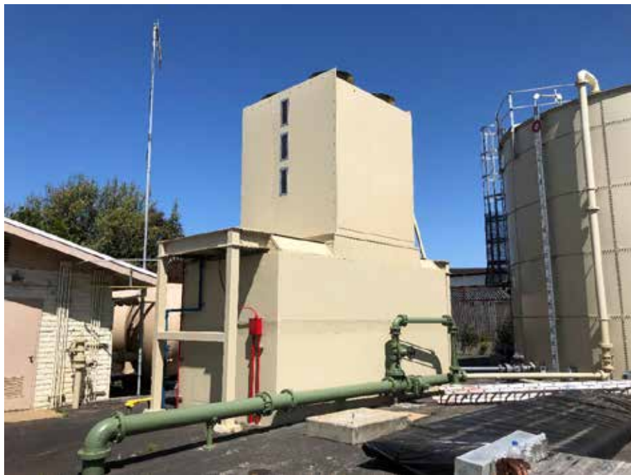
Exhibit 4. Aerator and Sump Pump, view looking northwest (IMG_0218).
