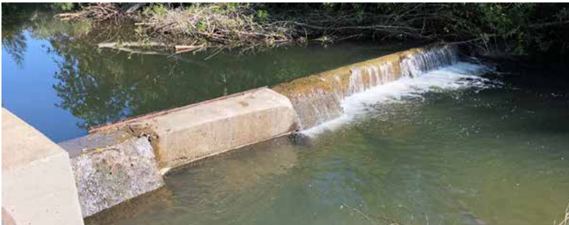
Exhibit 6. Tait Diversion, remaining section of the original concrete diversion dam, view looking north (IMG_0165).
