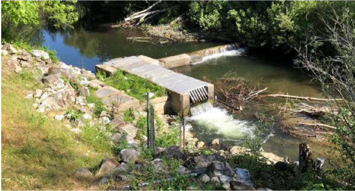
Exhibit 5. Tait Diversion, overview showing the 1983 intake in the foreground and the remaining section of the original concrete diversion dam stretching across the San Lorenzo, view looking north (IMG_0175).
