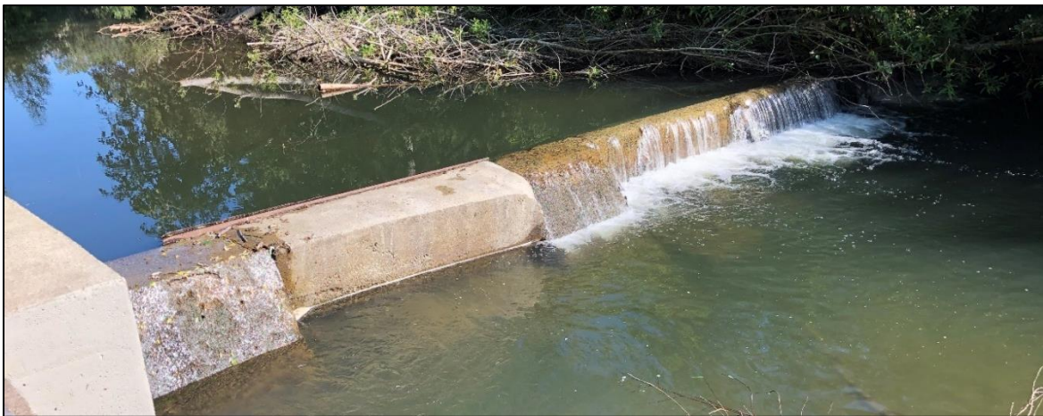
Exhibit 22. Tait Diversion, remaining section of the original concrete diversion dam, view looking north (IMG_0165).
