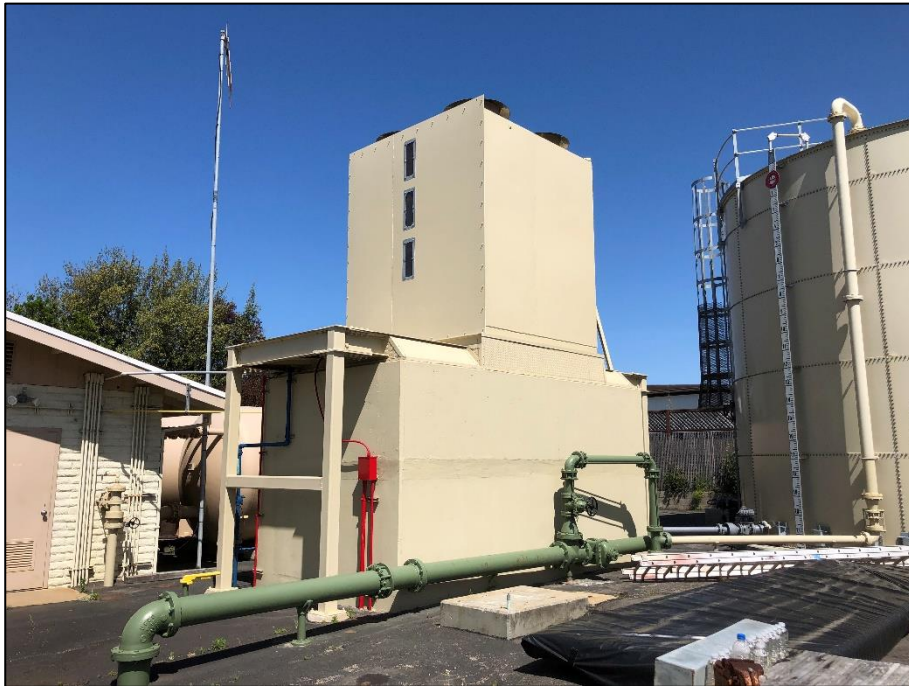
Exhibit 12. Aerator and Sump Pump, view looking northwest (IMG_0218).
