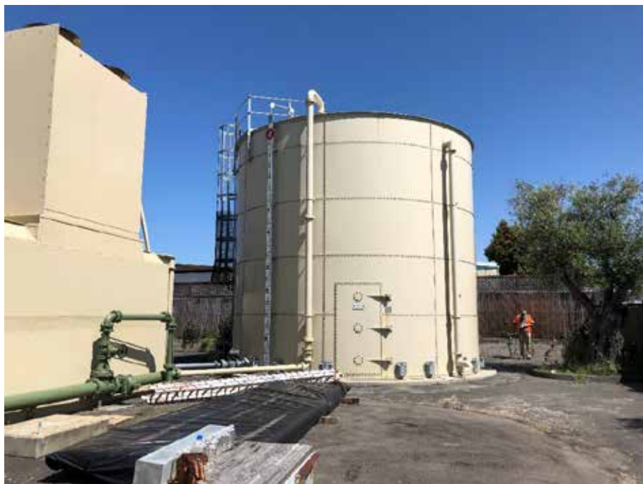
Exhibit 5. Wash Water Recovery Tank, view looking north (IMG_0219).
