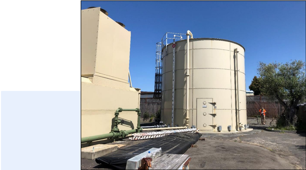
Exhibit 13. Wash Water Recovery Tank, view looking north (IMG_0219).
