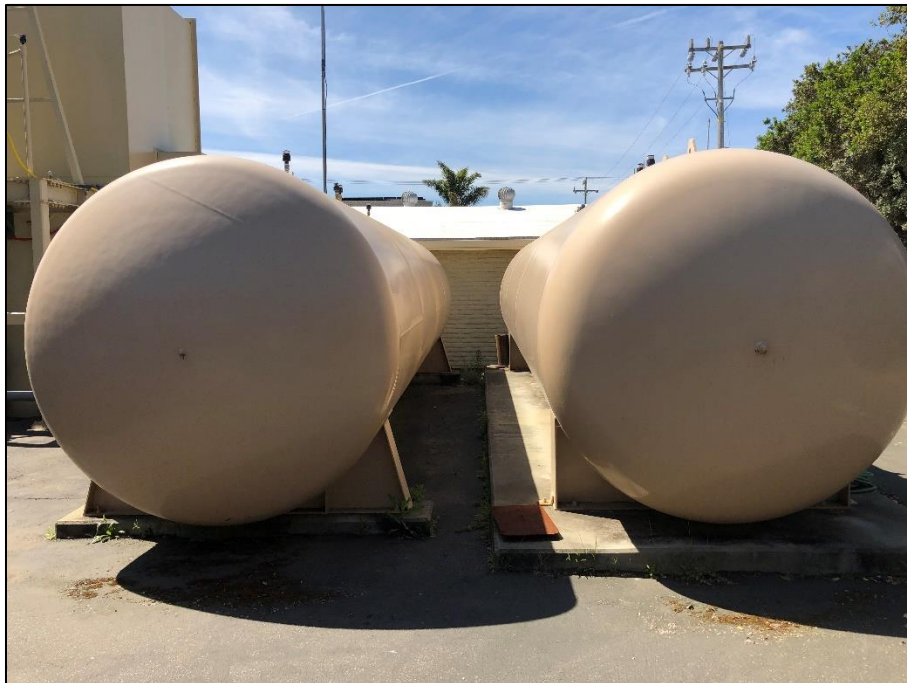
Exhibit 11. Two cylindrical pressure filters, view looking east (IMG_0220).
