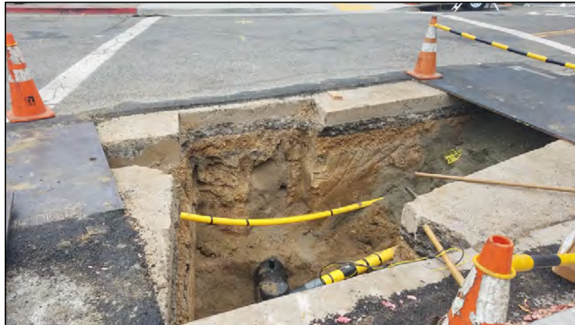
Figure 19. Utility trench at Adeline St and Harmon St. Note presence of trench sand, several layers of asphalt surface, and utilities 3-4 feet below ground surface.
