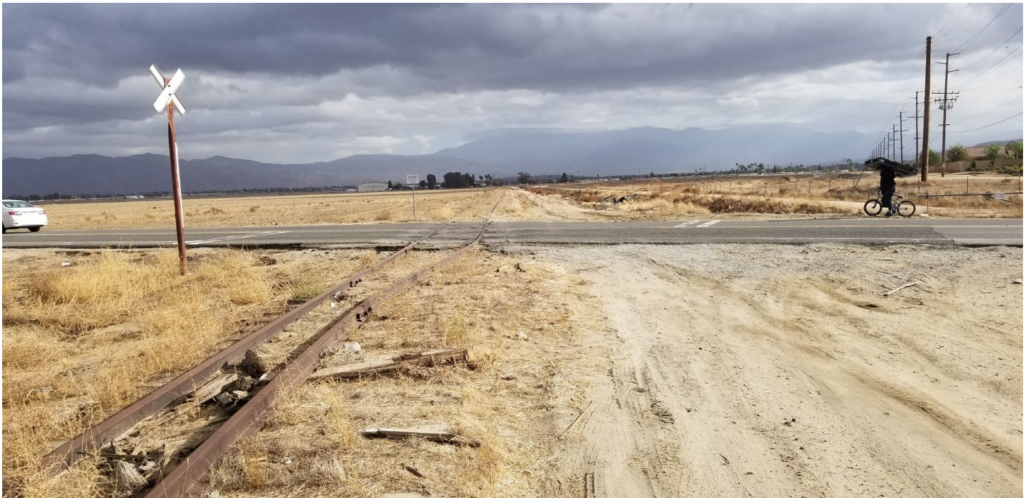
View east-northeast along south side of the tracks – note damaged rail and displaced ties.
