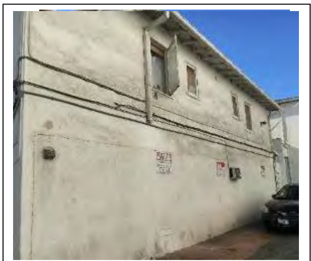
The rear structure at 1333 Ocean Avenue, which has been previously assessed for historical significance, is not identified in the City's HRI Update.
