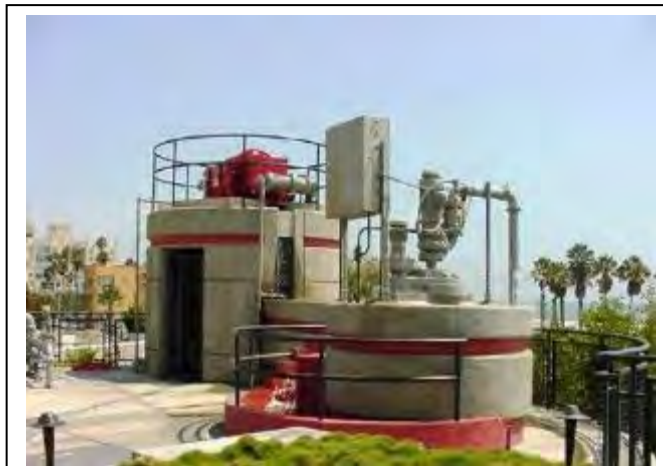
The SMURRF has the capacity to capture and treat approximately 0.5 MGD of urban runoff, contributing an average of 154 AFY of recycled water for non-potable use in the City.
