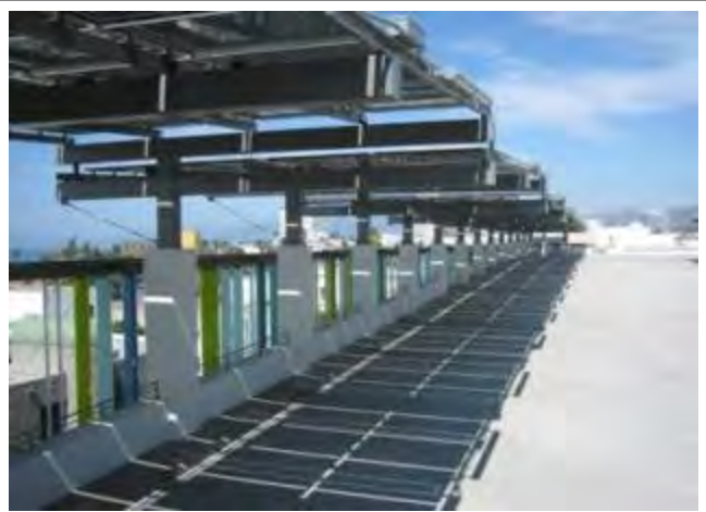
The City has installed a number of photovoltaic (PV) solar systems, including at public parking structures.
