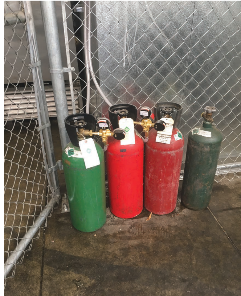
2) View of compressed gas cylinders observed at the rear of the Site restaurants.
