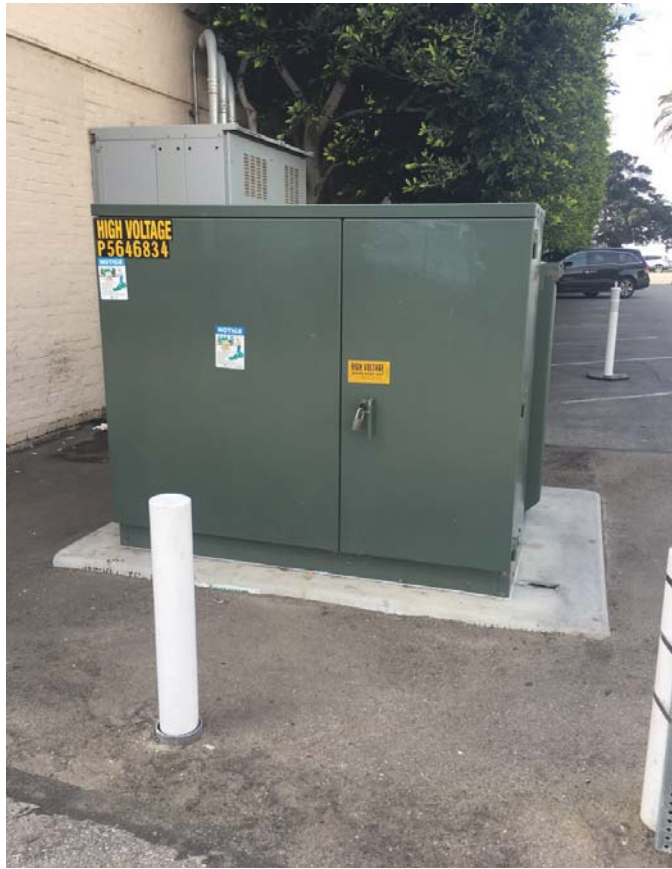
1) View of a transformer observed to be located at the Site.
