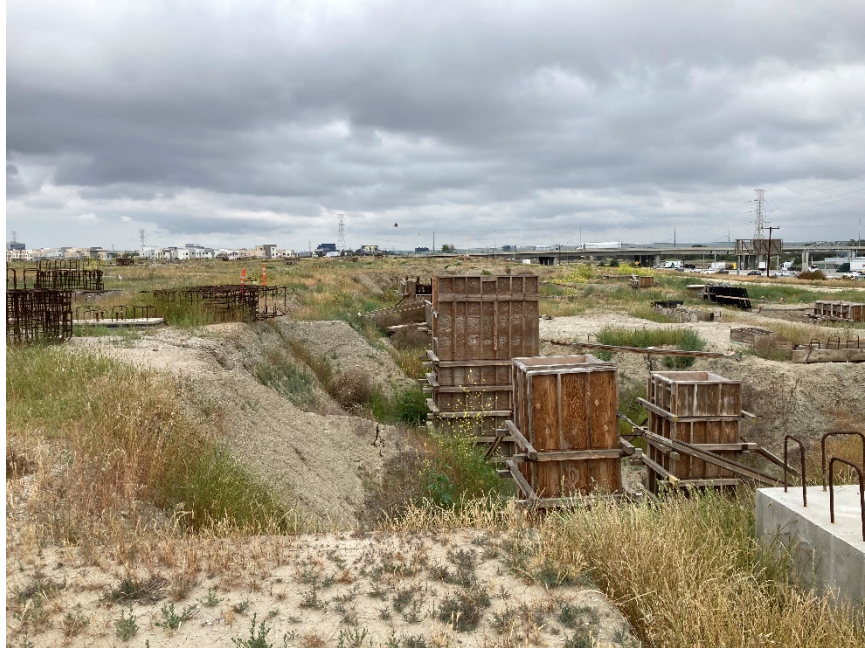
Site Photograph 7 – View of partially constructed structures and trenches in the eastern portion of the site. Photo taken facing north.
