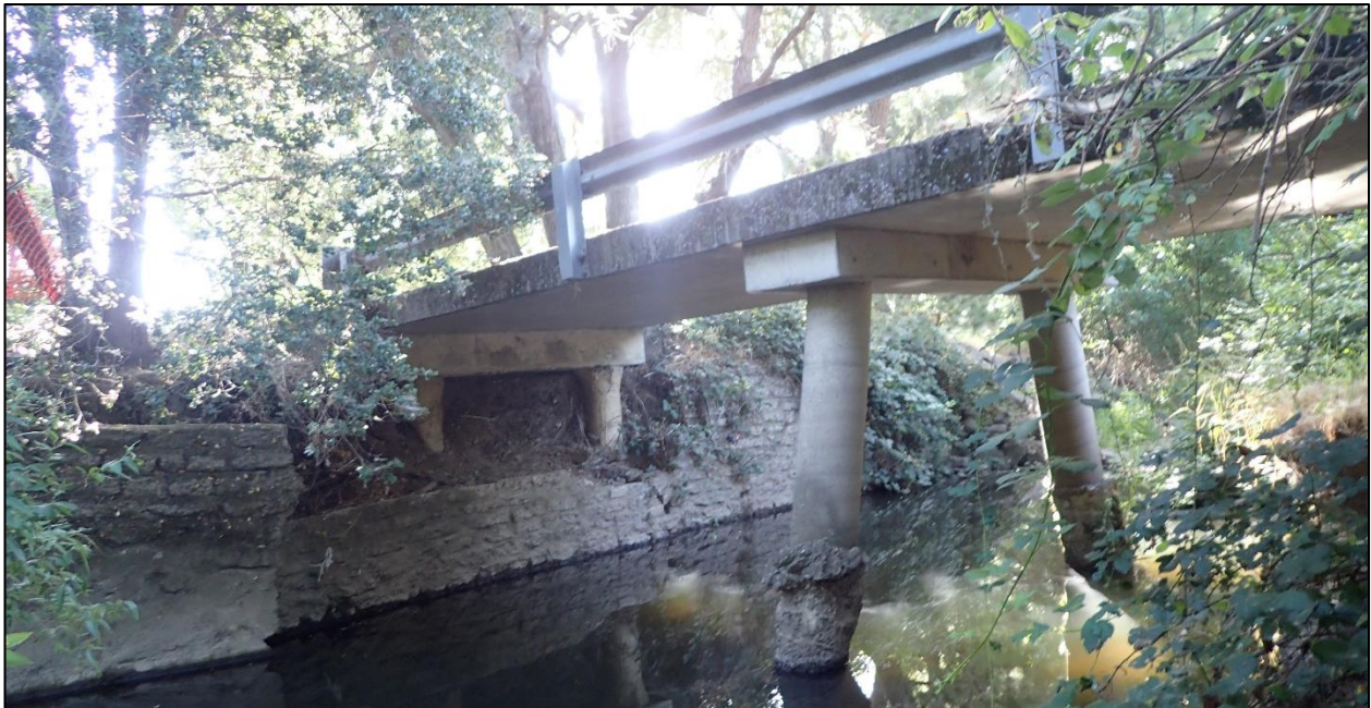
Photograph 4. Image shows the existing bridge that crosses Salvador Creek in the northern portion of the Study Area. View facing southeast. Photograph taken June 28, 2018.
