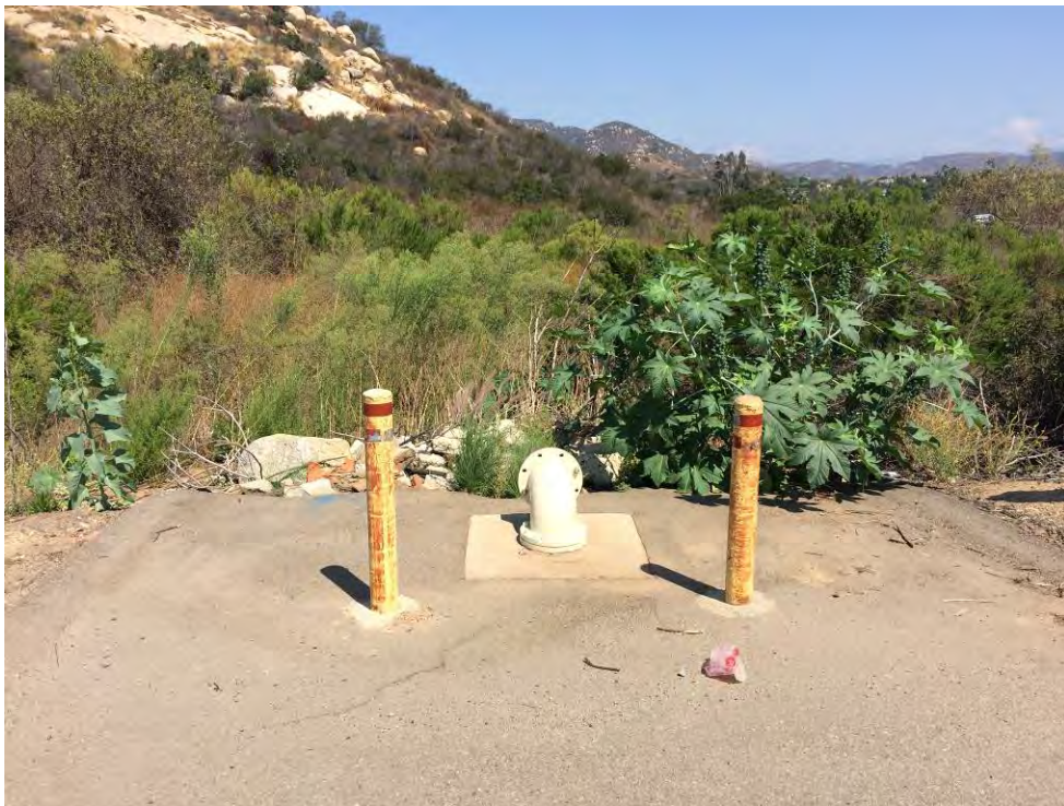
Photograph 12 – View looking at a water utility connection, located at the east-central region of the property, along the north side of N. Nutmeg Street.
