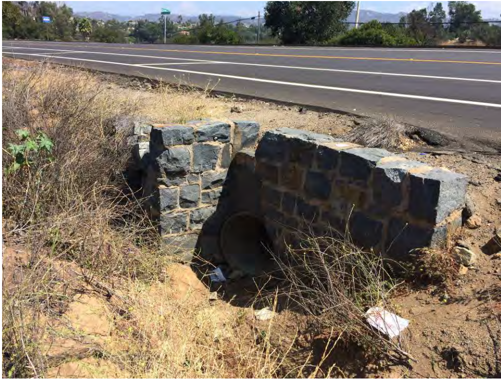
Photograph 11 – View of a storm drainage, located near the eastern perimeter of the property; along N. Centre City Parkway and north of N. Nutmeg Street.
