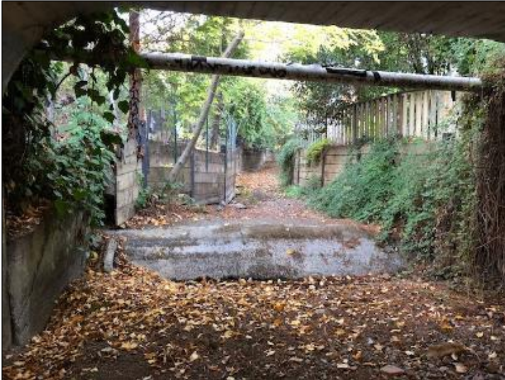
View 2. View upstream from under the Shady Lane bridge of abandoned concrete sewer line/casing.
