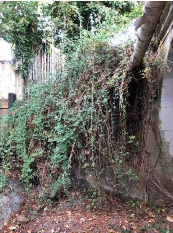
View 4. View of bank at northwest abutment of the Shady Lane bridge crossing, with heavy ivy and blackberry cover on bank and growing into Monterey pine near top of bank.
