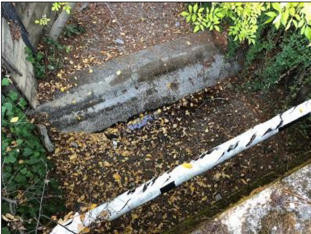
View 6. View from above of the concrete casing across Ross Creek upstream of the Shady Lane bridge.
