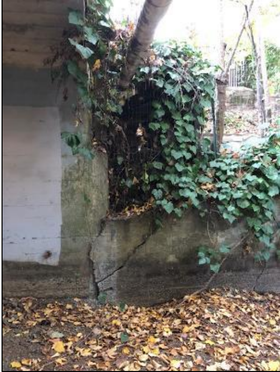
View 3. View of bank at southwest abutment of the Shady Lane bridge crossing, with heavy ivy cover.
