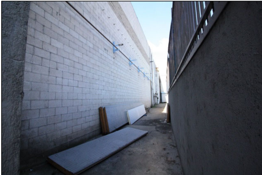
Rear (east) elevation with concrete block exterior and new concrete wall to the east, view north
