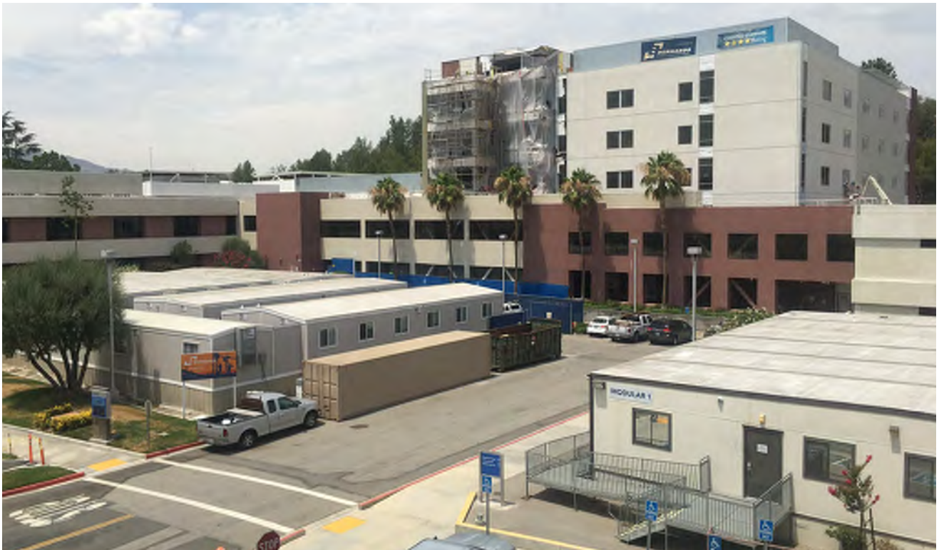
Inpatient Building No. 1 (IP-1) under construction in 2018 when the Notice of Preparation for this SEIR was released.
