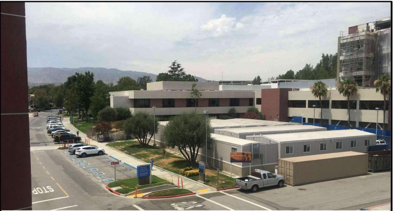
Conditions at Lot D and Lot H in 2018, at the time that the Notice of Preparation was issued.
