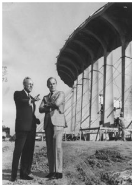
The Forum under construction, with Jack Kent Cooke and Charles Luckman, 1967. ( Herald Examiner Collection, LAPL )
