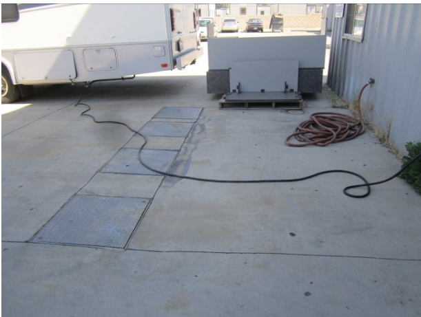
29. View to north of the three-stage subsurface interceptor located west of the Maintenance Building
