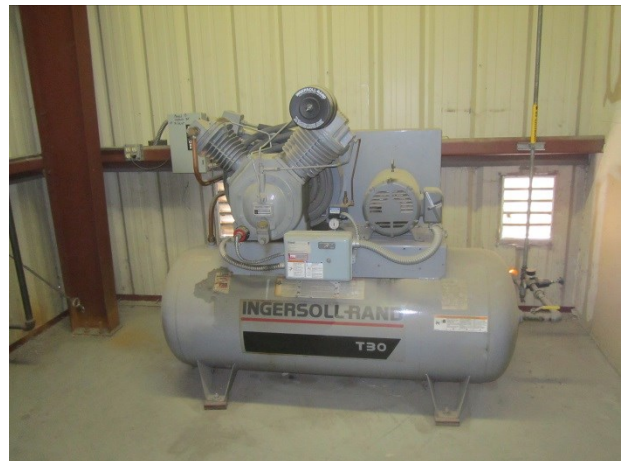
30. Compressor located within the Maintenance Building
