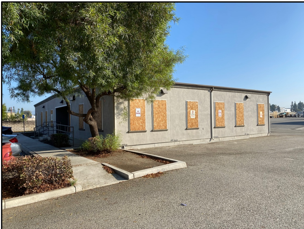
Plate 3.2-2: View of the boarded-up office building in the northwest portion of the project, facing northeast.
