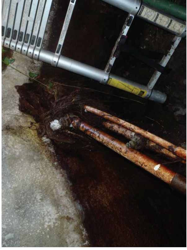
Old in-operable valve on apparent low-level discharge pipe at portal
