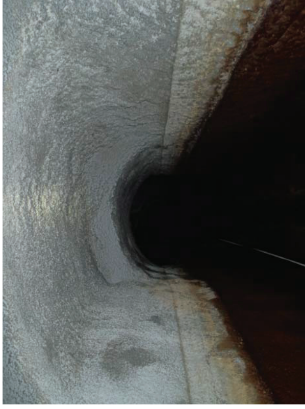
Curve area about 25' into tunnel, tunnel height lowers then raises at apparent transition from cut/cover to mined tunnel location (old portal?)
