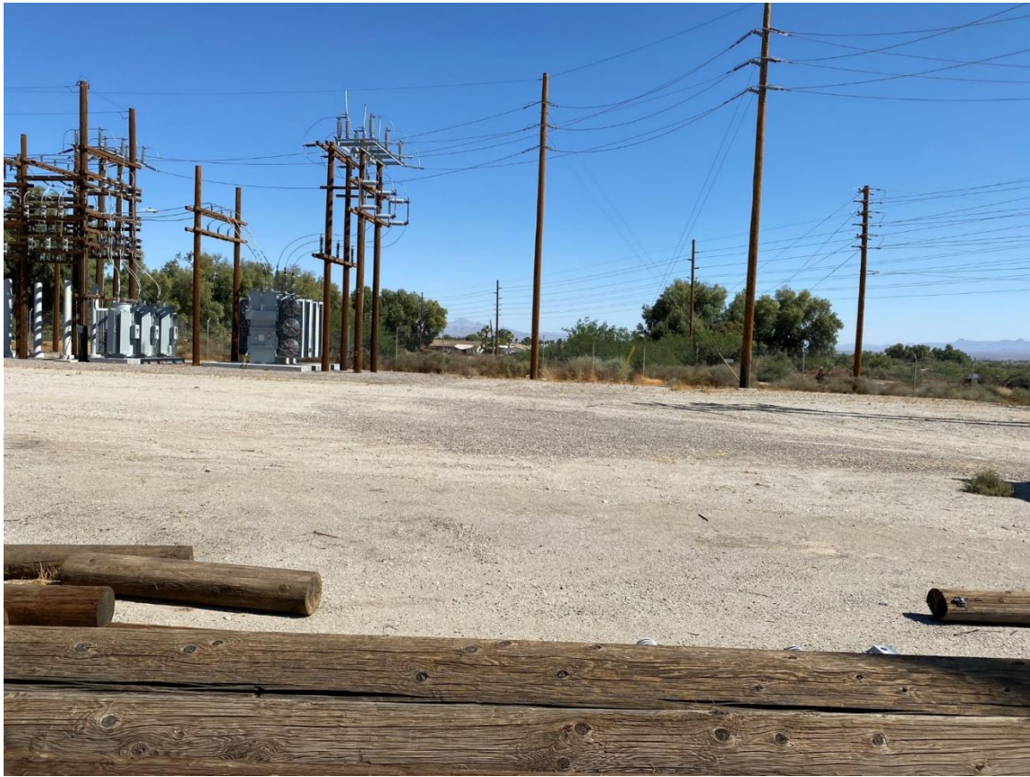
Photo 3 – Southern portion of Project site, facing North. Near the center of the sub-station fencing, adjacent to the proposed access road.
