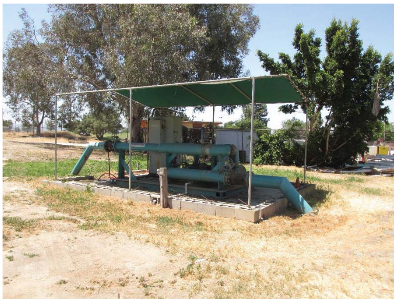
Figure 22. Mechanical Equipment, Image No. IMG_5747.
