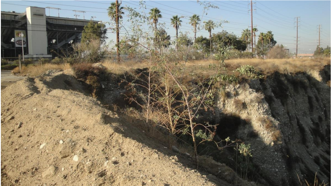
Photograph No. 3: Scarp north of Live Oak Avenue, Irwindale Raceway in left background – View WSW
