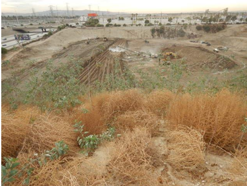
Photograph No. 7: Active IDEFO on the southeast portion of the site. 605 freeway on left, bridge is Live Oak Ave. - view South
