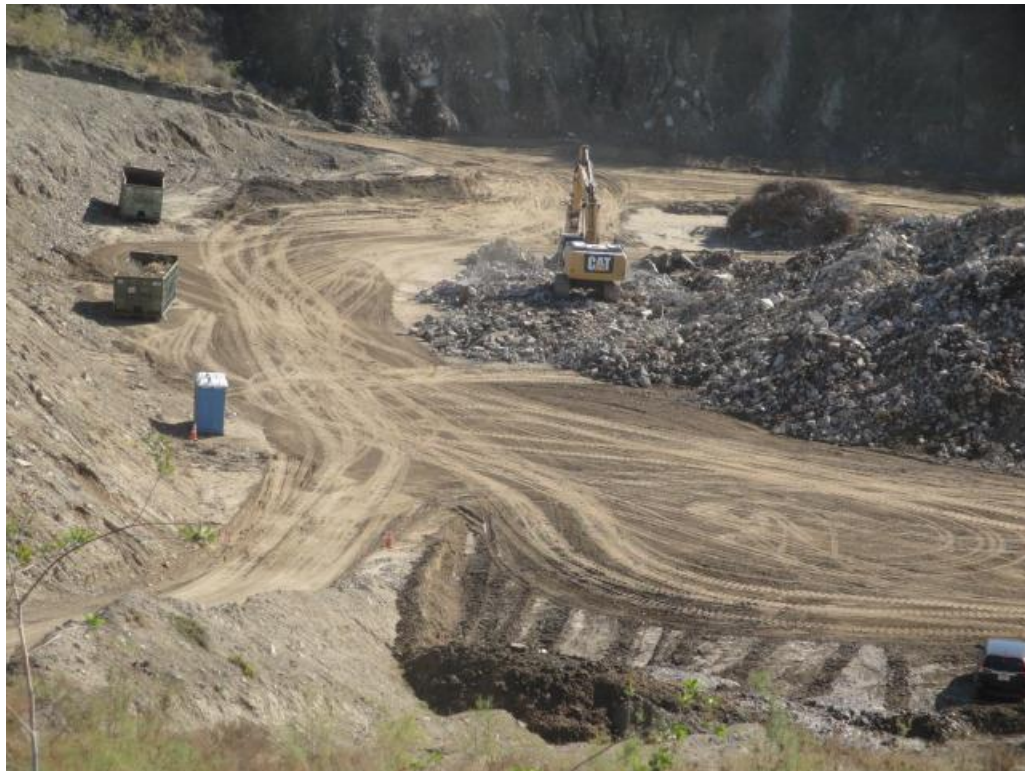
Photograph No. 2: IDEFO operation in east quarry, bins for reject metal and trash – view East
