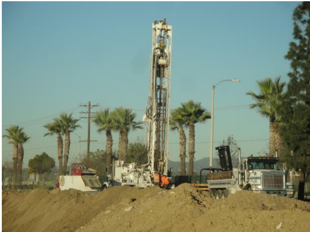
Photograph No. 12: Water supply well drilled (2017) just south of Arrow Highway – view NW
