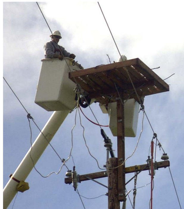
A PG&E crew installs a nest platform near Clear Lake. Nest platforms reduce outages and are preferred by large birds, such as ospreys.
