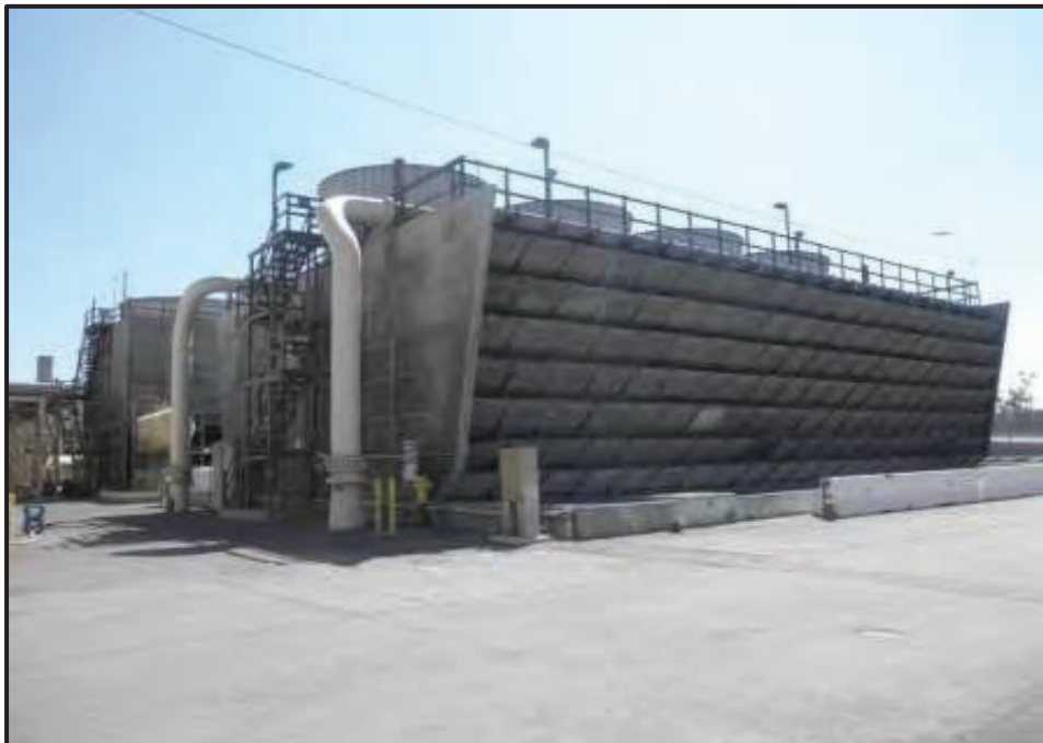
Photograph 12. Cooling Tower No. 2 (No. 1 in background), View Looking Southeast (Photo by J. Terry).
