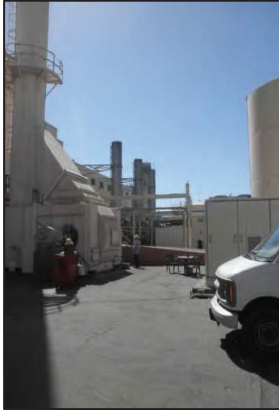
Photograph 6. Boiler Stacks (Boilers 1 and 2 Center Rear of Photograph; Boiler 3 to Left), View Looking South. (Photo by J. Terry).
