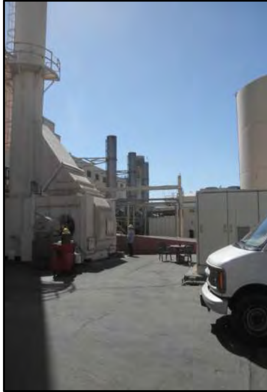
Photograph 6. Boiler Stacks (Boilers 1 and 2 Center Rear of Photograph; Boiler 3 to Left), View Looking South. (Photo by J. Terry).
