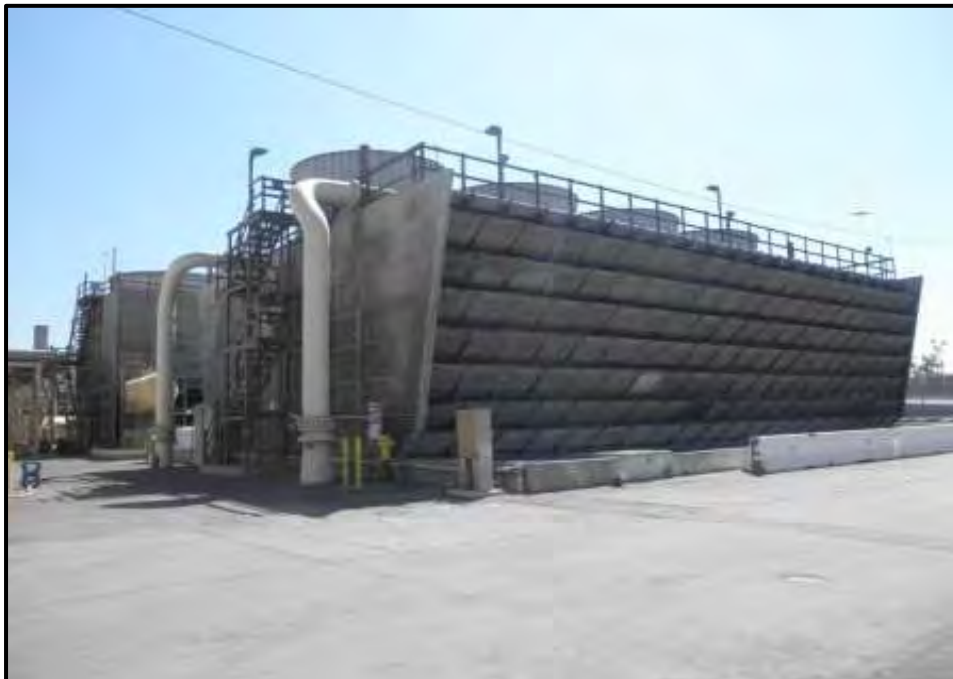
Photograph 12. Cooling Tower No. 2 (No. 1 in background), View Looking Southeast (Photo by J. Terry).
