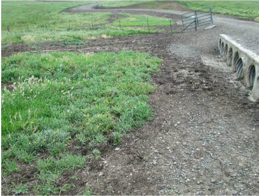
Photo 1. Field 18 with disturbed soil near culvert dominated by yellow starthistle and Italian thistle, view east. April 12, 2016.
