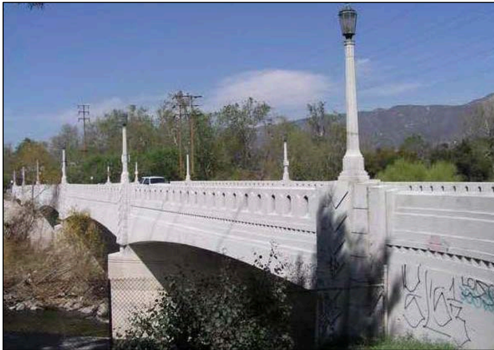
Photograph 2. Riverside Boulevard over Los Angeles River (Bridge No. 53C1298), note chevron detailing above each pier, detail at bottom of rail, and street lights. 40
