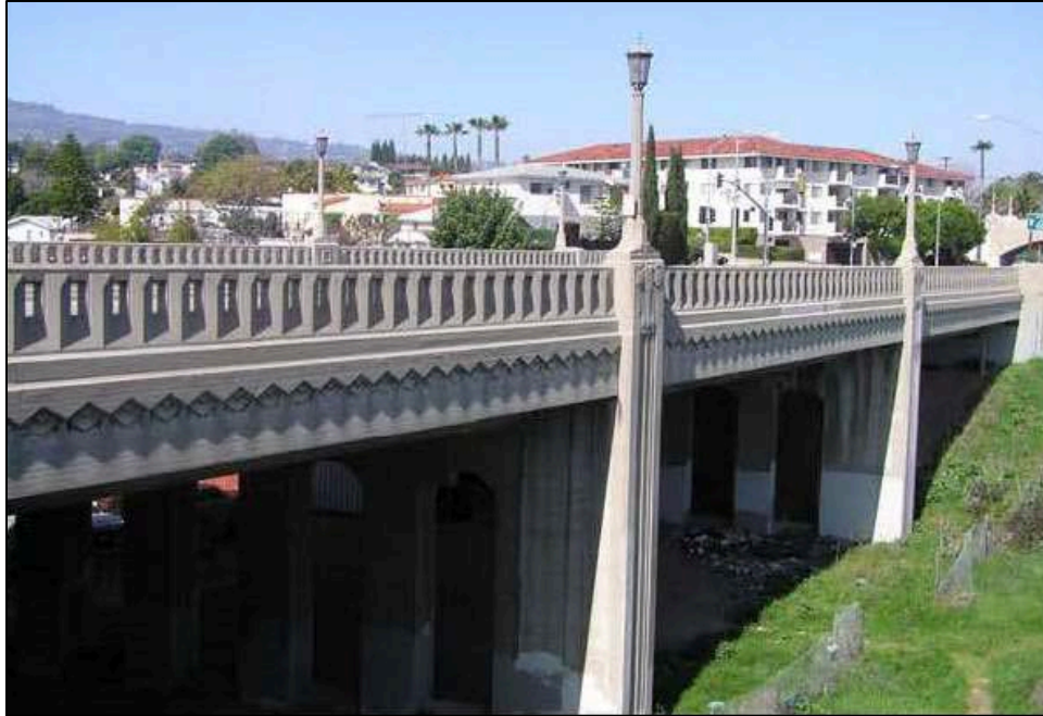
Photograph 1. Gaffey Street Bridge, note the detailing on the supporting piers, the zig zag across the bottom of the rails, and the light posts (Bridge No. 53 0397Y). 39
