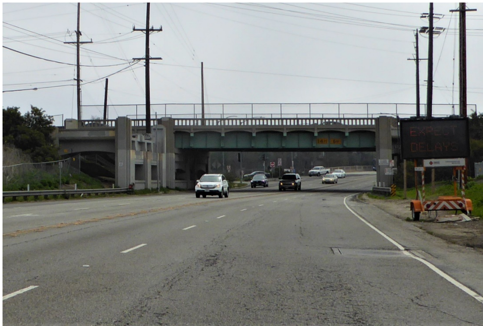
Photograph 1: Pacific Electric / SR 1 bridge approach spans; camera facing south, Culver Boulevard overcrossing in background, March 29, 2018.
