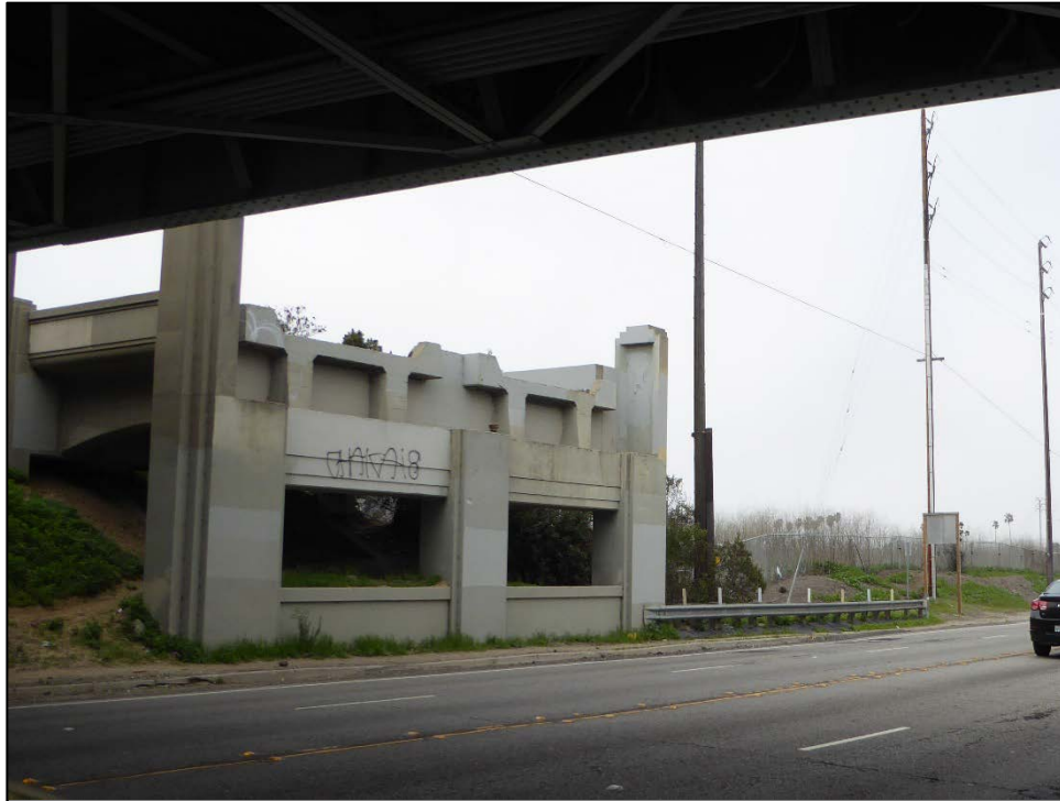
Photograph 2: Pacific Electric / SR 1 bridge approach span; camera facing northwest showing supports for rail beds, March 29, 2018.
