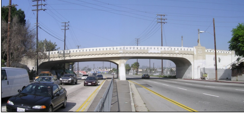
Photograph 3. West Boulevard over Venice Boulevard (Bridge No. 53C1380) note decoration at end pier. 41
