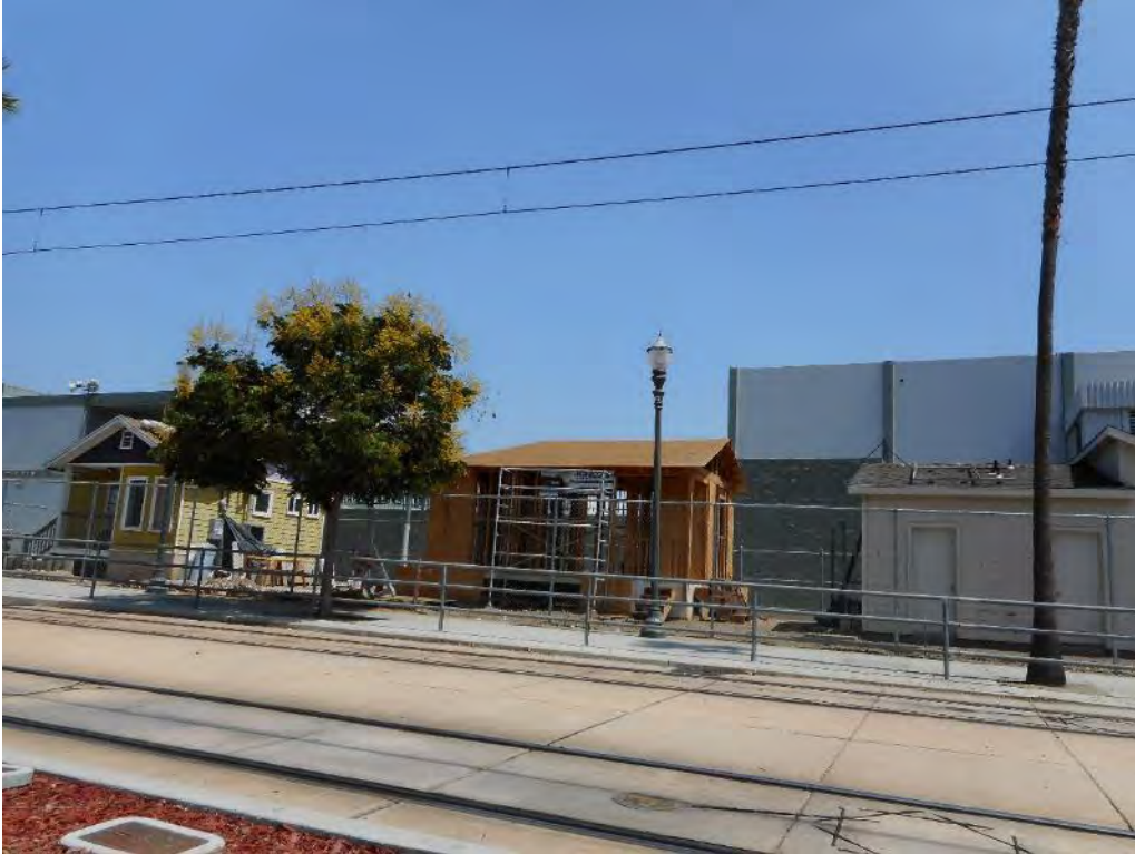
105. Laurel Gymnasium & Willow Hall with outdoor class construction area along Flower St
