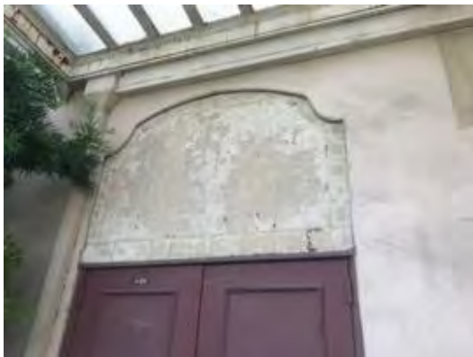
Detail of missing decoration above doors
