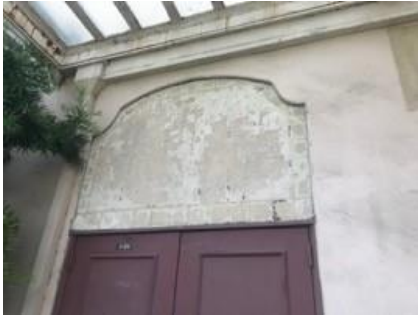
Detail of missing decoration above doors
