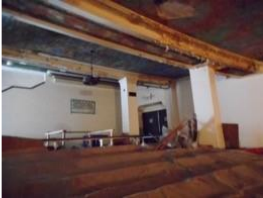
Entrance into main assembly area and area under balcony and stairs to balcony on rear wall, 2018
