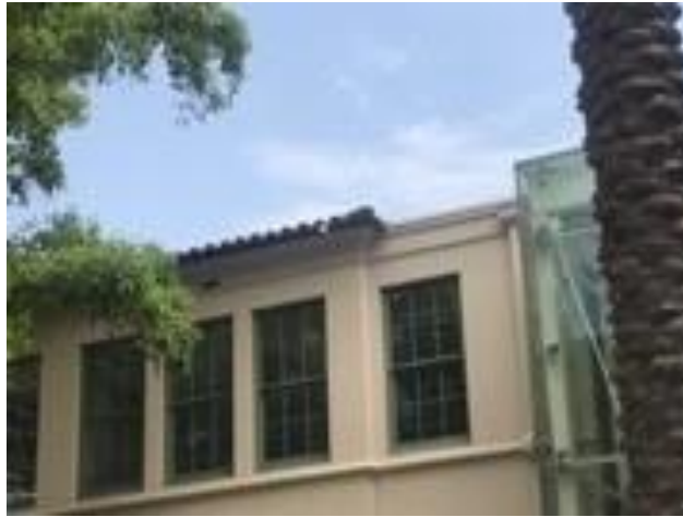
Building detail of West Classroom Building where it meets the new south entrance to Magnolia Hall
