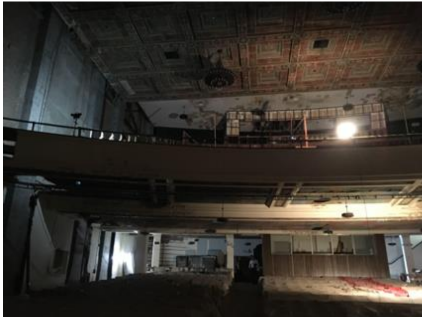
Looking to the rear of theater, ceiling above main floor has decorative painting, ceiling above balcony does not have decorative painting, 2018
