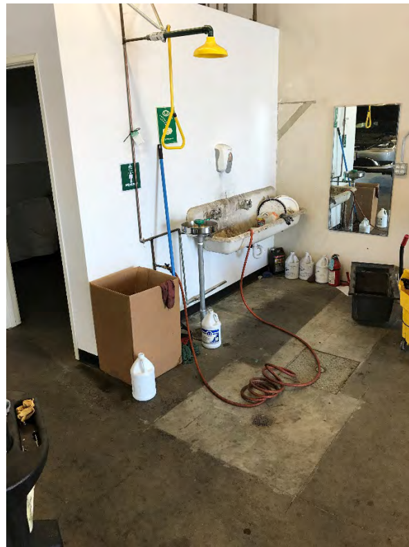
Emergency wash station and floor drain in the automotive maintenance building
