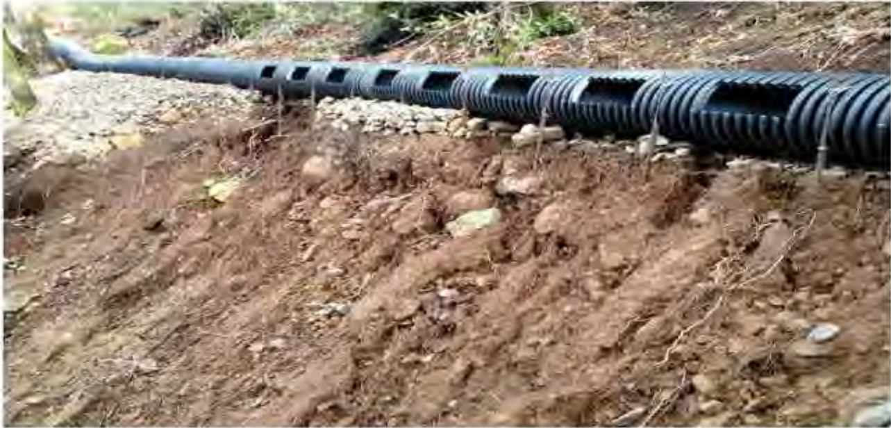
Figure 13 Feb. 2, 2012 Level Spreader Failure into Burton Creek from Cliff Family Vineyard
