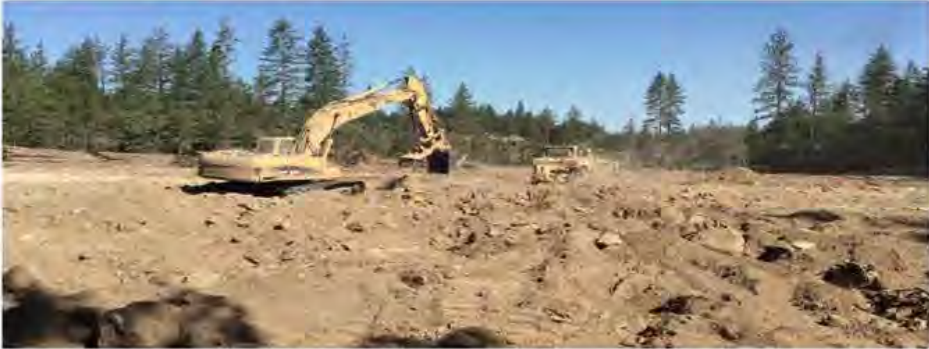
Figure 6 Typical vineyard construction scene Las Posadas Rd Bremer Family Winery Vineyard. Note equipment utilized in rock clearing.
