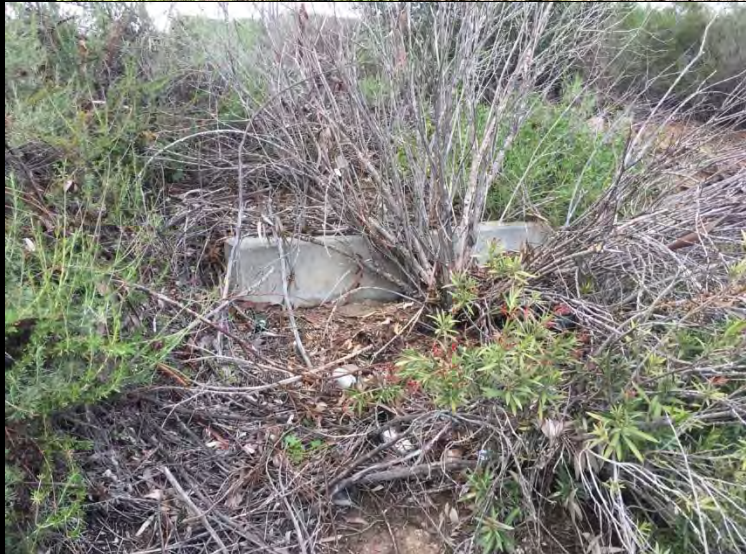
Representative Photograph 2. Facing E. Blocked outfall
