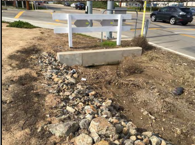
Representative Photograph 3. Facing N. Blocked outlet
