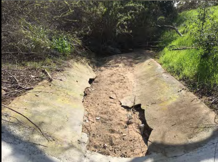
Representative Photograph 3. Facing NW. Portions of concrete is broken and in need of repairs.
