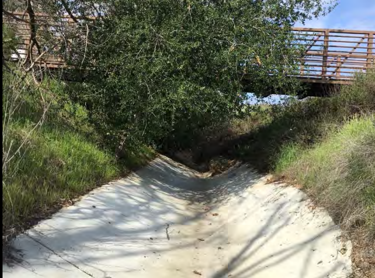
Representative Photograph 2. Facing NW. Concrete channel at upstream end as it flows under a pedestrian bridge crossing.
