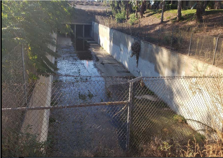
Representative photo of the southern section of the maintenance site, a concrete-lined channel.
