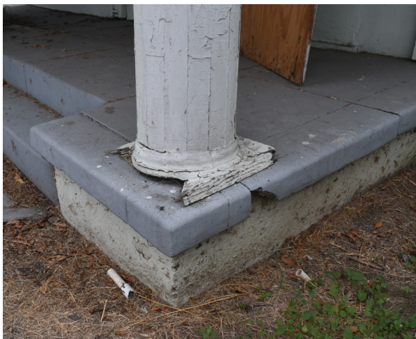
Figure 25: Damaged column base.
