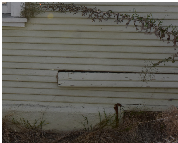
Figure 17: Damaged clapboard siding.
