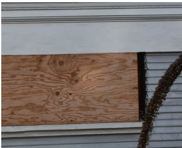
Figure 19: Original wood window, missing trim.
