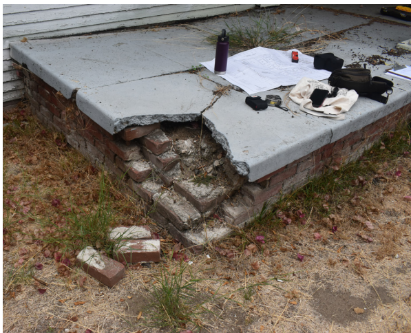
Figure 22: Damaged front porch.
