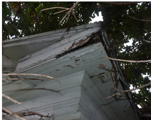
Figure 23: Damaged boxed eaves.
