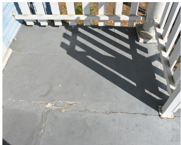
Figure 15: Cracked concrete front porch.
