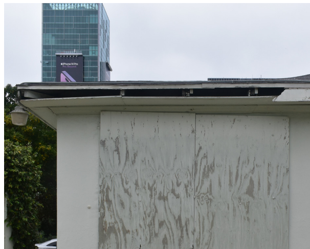
Figure 26: Missing fascia board on boxed eaves.
