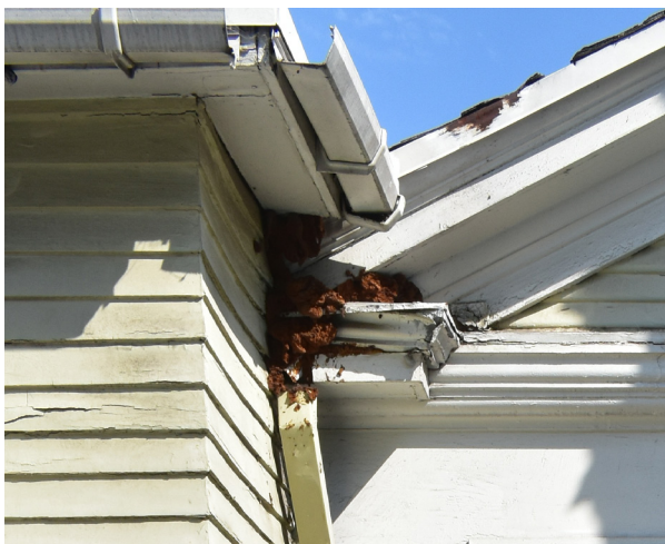
Figure 16: Damaged cornice return and plain frieze.
