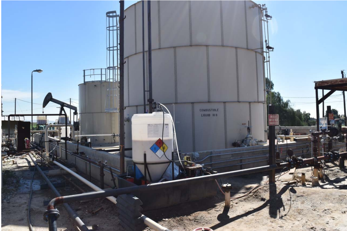
41. Brea Production Unit and Olinda Tank Farm located in the central area of the northern portion of the 165-Acre Parcel.
