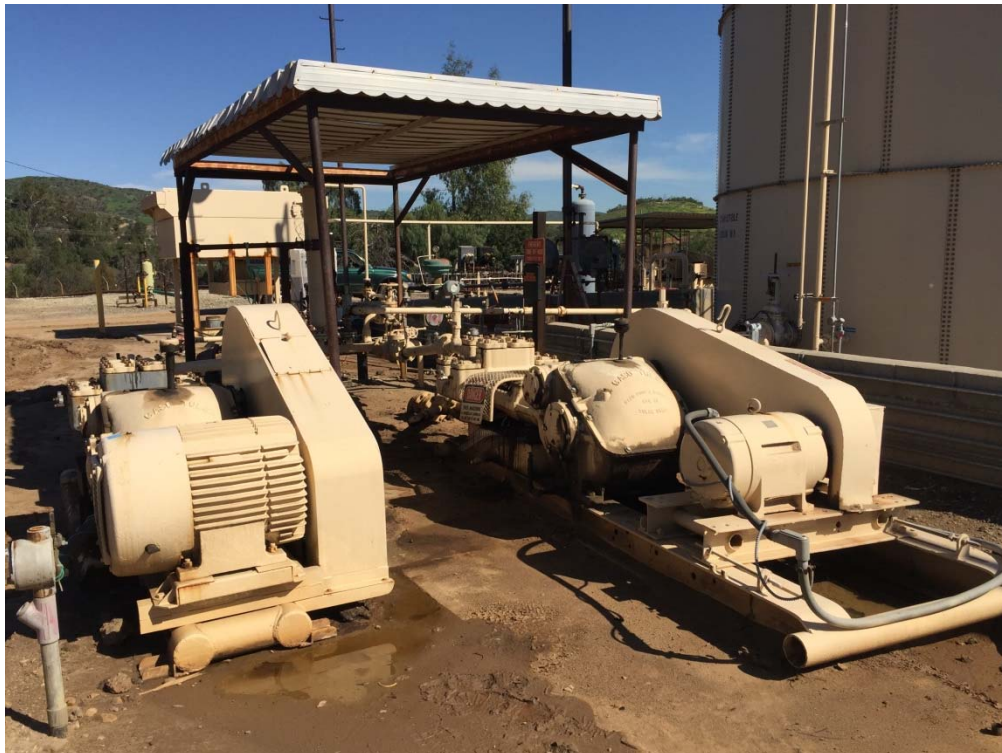
46. Brea Production Unit and Olinda Tank Farm located in the central area of the northern portion of the 165-Acre Parcel.
