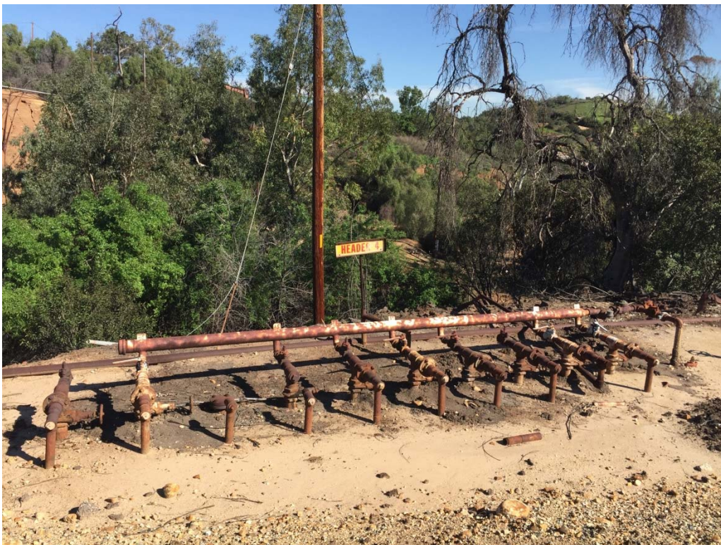
38. Typical manifold header located in the northern and central portions of the 165-Acre Parcel.
