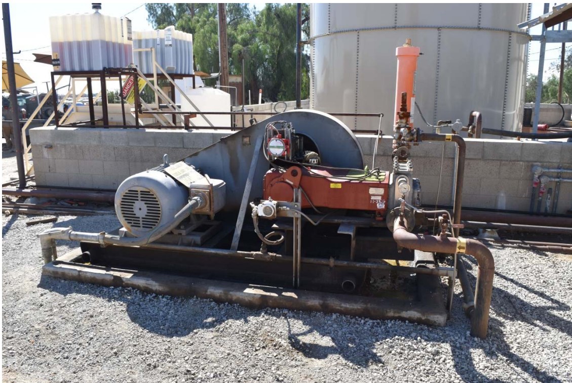
42. Brea Production Unit and Olinda Tank Farm located in the central area of the northern portion of the 165-Acre Parcel.
