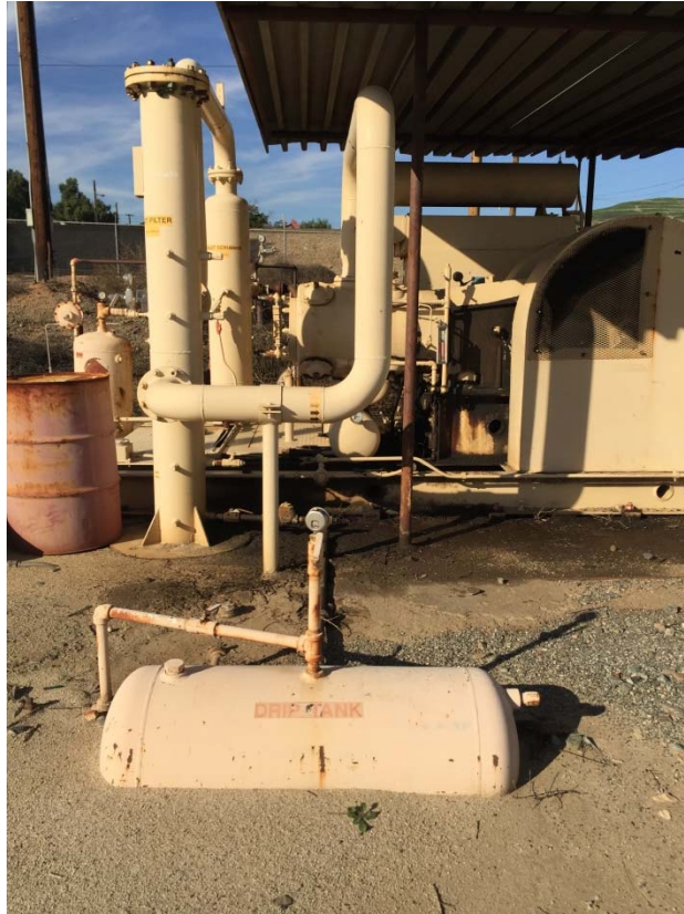
23. Vapor recovery system located in the north central area of the southern portion of the 100-Acre Parcel.
