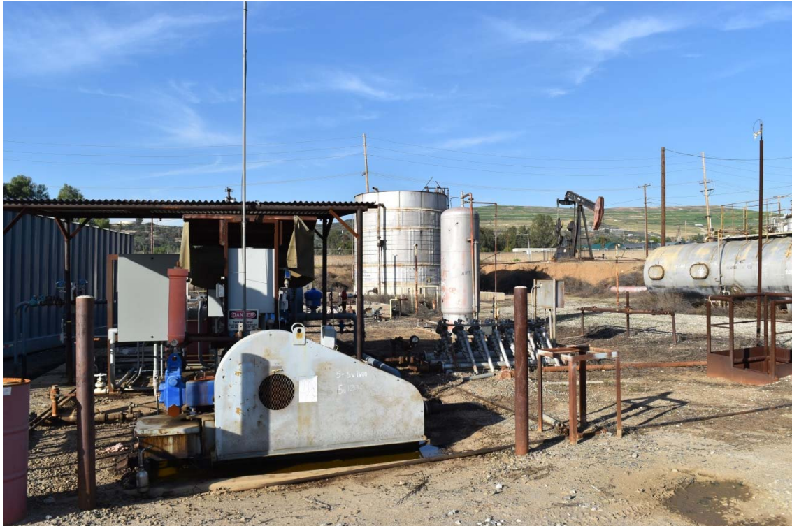
29. Dehydration Unit located in the north central area of the southern portion of the 100-Acre Parcel.
