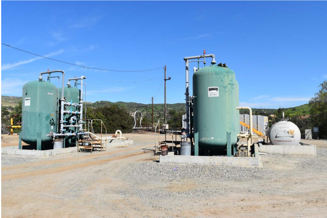
47. Carbon filtration area located in the central area of the northern portion of the 165-Acre Parcel to the south of the Brea Production Unit and Olinda Tank Farm.
