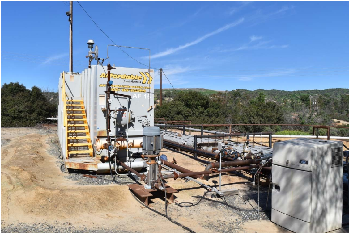
50. Carbon filtration area located in the central area of the northern portion of the 165-Acre Parcel to the south of the Brea Production Unit and Olinda Tank Farm.
