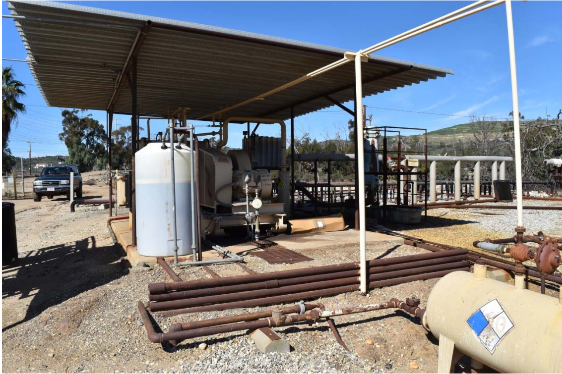
43. Brea Production Unit and Olinda Tank Farm located in the central area of the northern portion of the 165-Acre Parcel.
