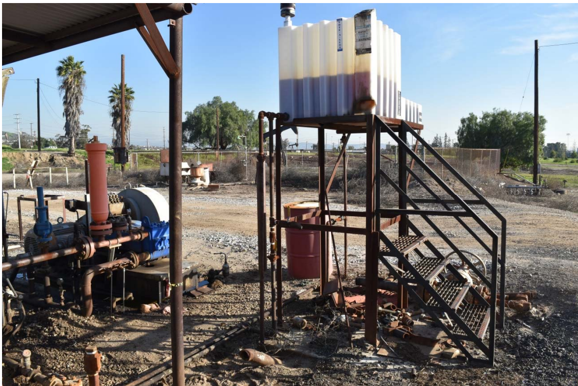
32. Dehydration Unit located in the north central area of the southern portion of the 100-Acre Parcel.
