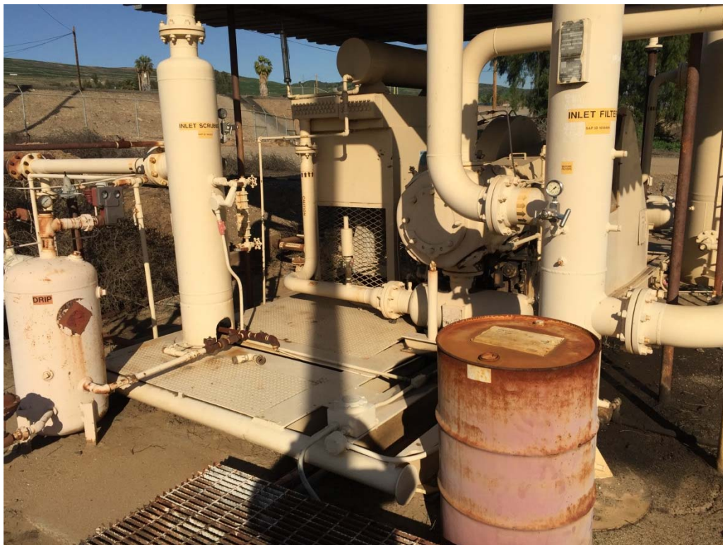
22. Vapor recovery system located in the north central area of the southern portion of the 100-Acre Parcel.
