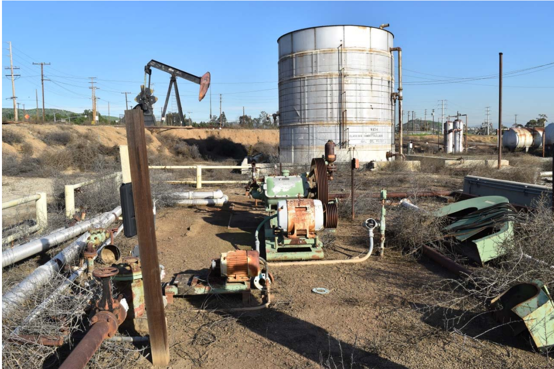
25. Dehydration Unit located in the north central area of the southern portion of the 100-Acre Parcel.
