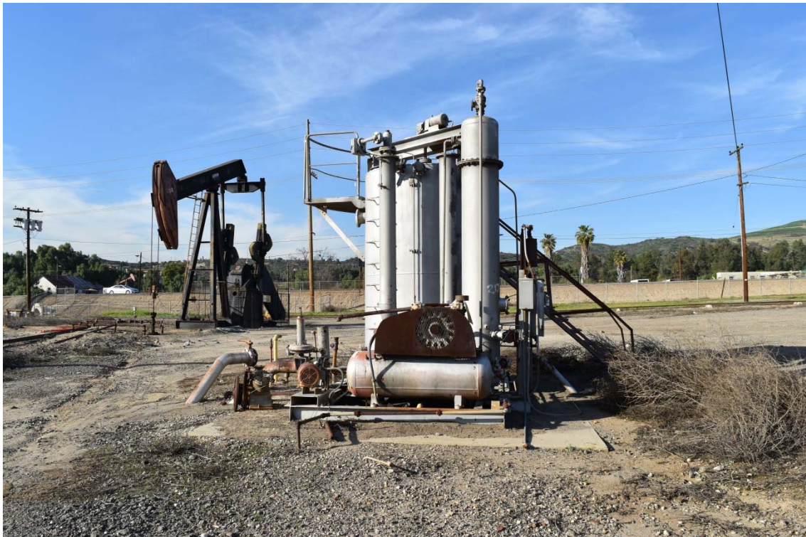
28. Dehydration Unit located in the north central area of the southern portion of the 100-Acre Parcel.
