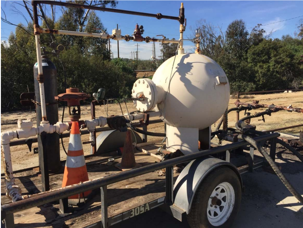
37. Portable well testing trailer located in the northern portion of the 165-Acre Parcel.
