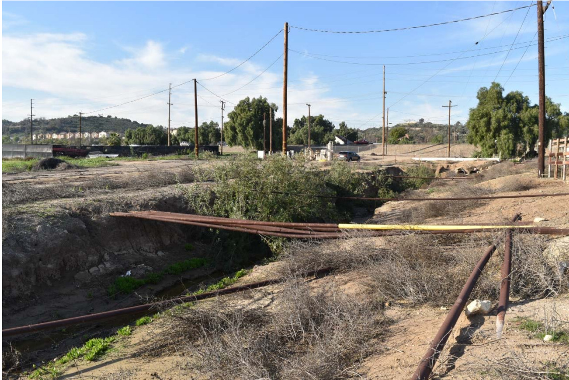
17. Oil well field pipelines suspended over the drainage channel in the southern portion of the 100-Acre Parcel.
