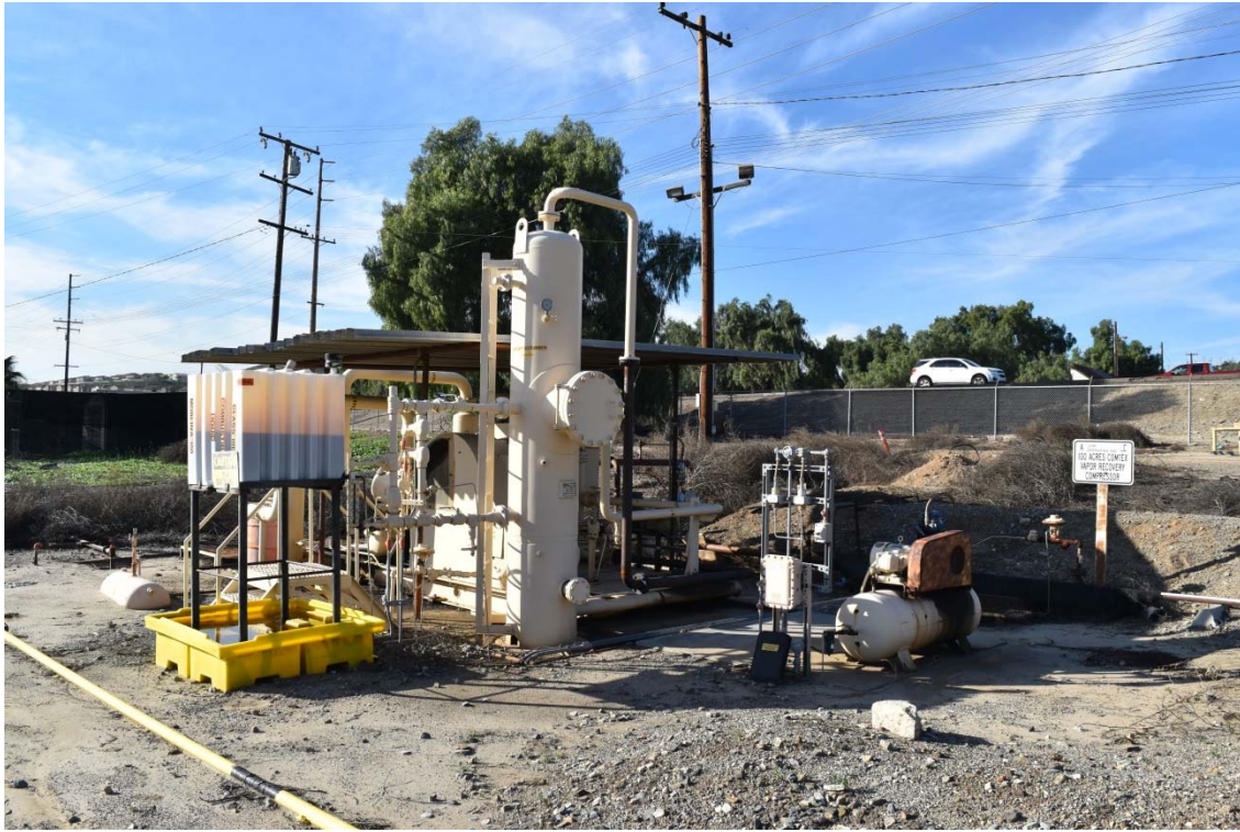
18. Vapor recovery system located in the north central area of the southern portion of the 100-Acre Parcel.
