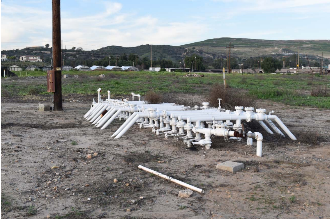
33. Typical manifold located on the southern portion of the 100-Acre Parcel.
