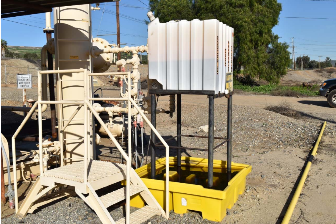
19. Vapor recovery system located in the north central area of the southern portion of the 100-Acre Parcel.
