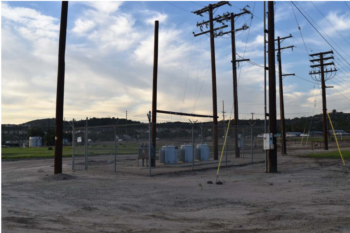
34. Transformers located in the central area of the southern portion of the 100-Acre Parcel.
