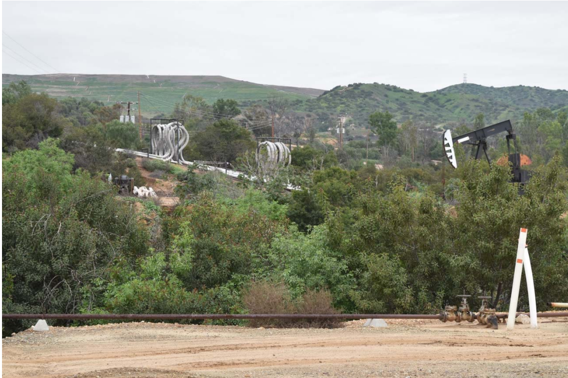
39. Steam pipes located in the northern and central portions of the 165-Acre Parcel.
