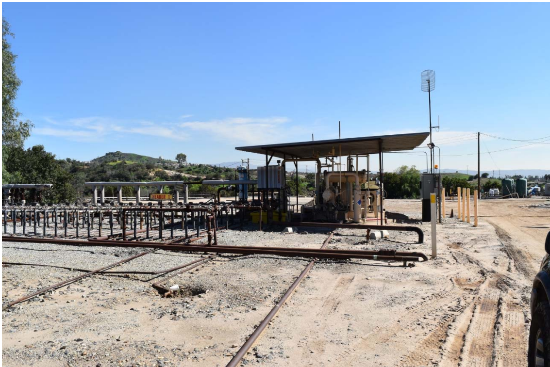
44. Header and compressor station in Brea Production Unit and Olinda Tank Farm located in the central area of the northern portion of the 165-Acre Parcel.
