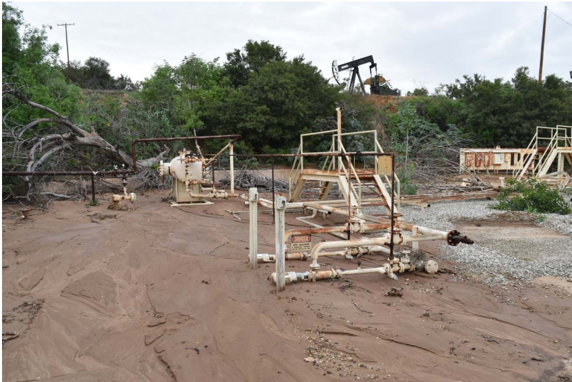
52. Former tank farm location in the south central portion of the 165-Acre Parcel.
