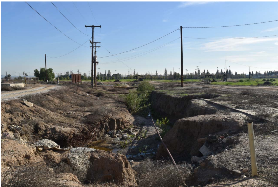
16. Typical drainage channel through the central area of the southern portion of the 100-Acre Parcel.
