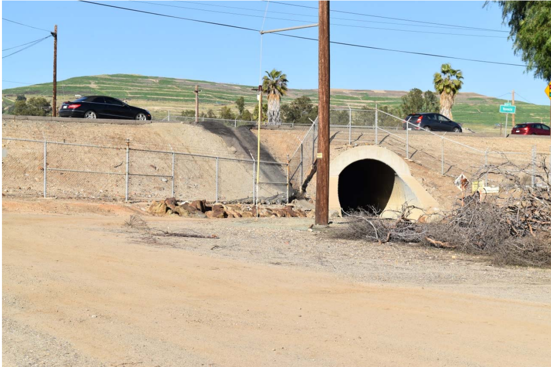
15. Drainage channel conduit under Lambert Road from the northern portion of the 100-Acre Parcel connecting to the southern portion of the 100-Acre Parcel.
