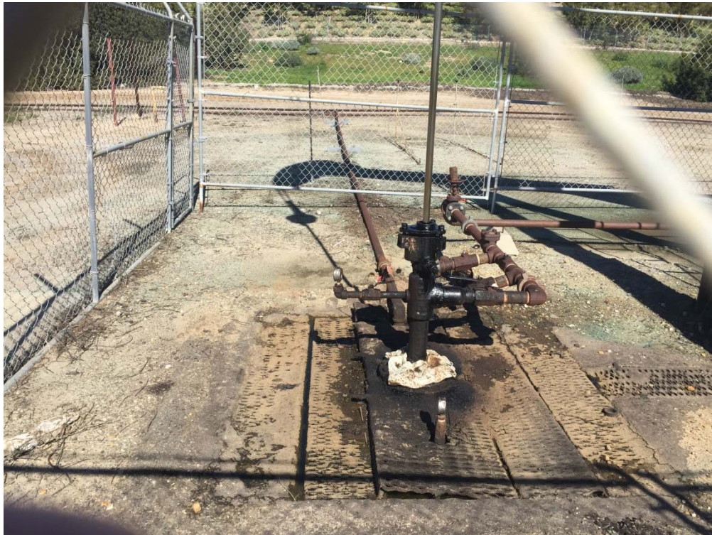
4. Typical oil well head of oil well located on the northern portion of the 100-Acre Parcel.
