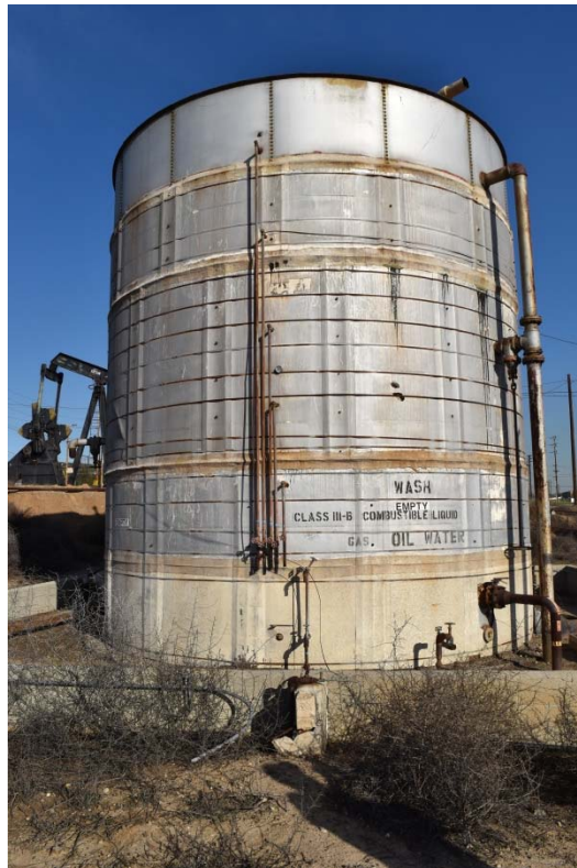
26. Dehydration Unit located in the north central area of the southern portion of the 100-Acre Parcel.
