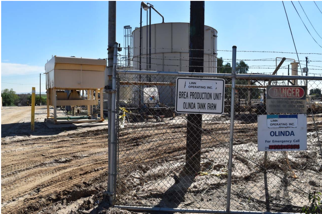
40. Brea Production Unit and Olinda Tank Farm located in the central area of the northern portion of the 165-Acre Parcel.
