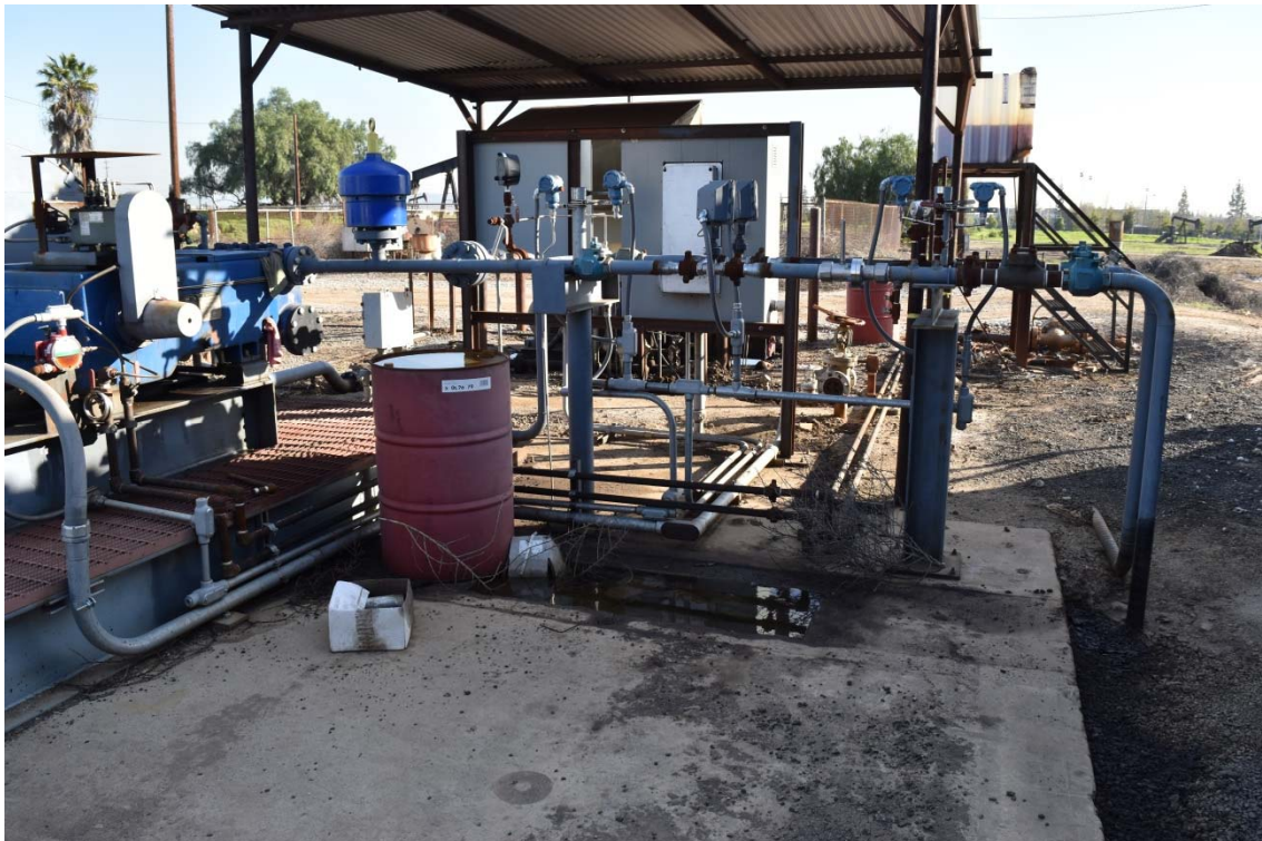
30. Dehydration Unit located in the north central area of the southern portion of the 100-Acre Parcel.
