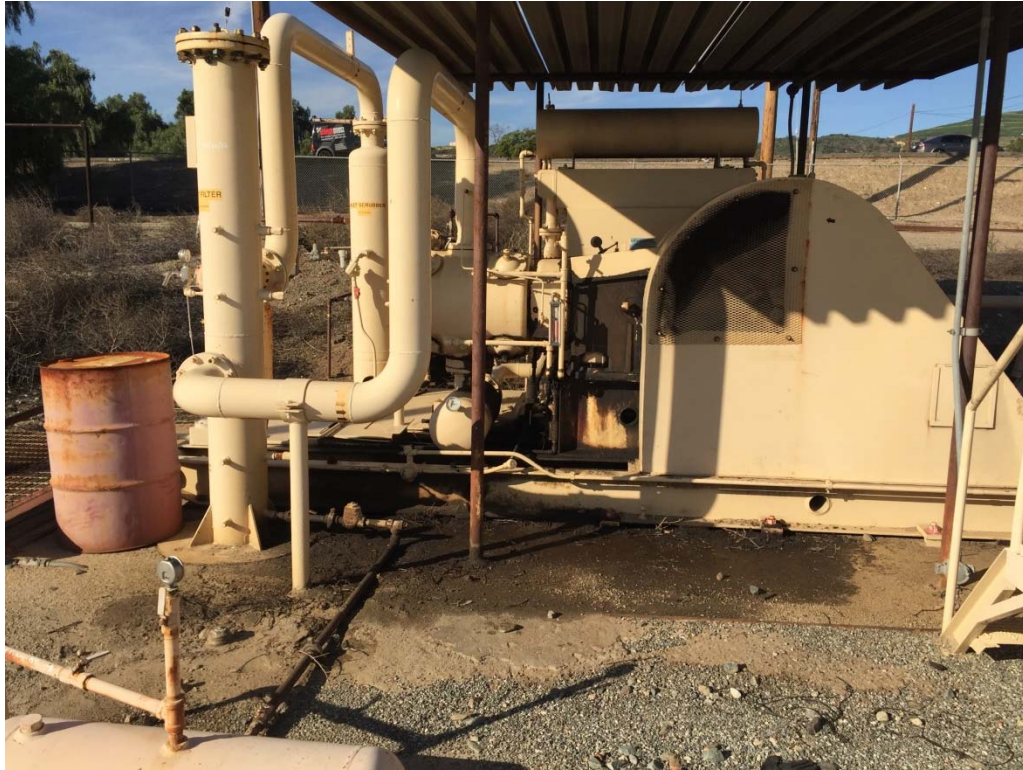
21. Vapor recovery system located in the north central area of the southern portion of the 100-Acre Parcel.
