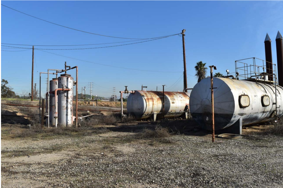
27. Dehydration Unit located in the north central area of the southern portion of the 100-Acre Parcel.
