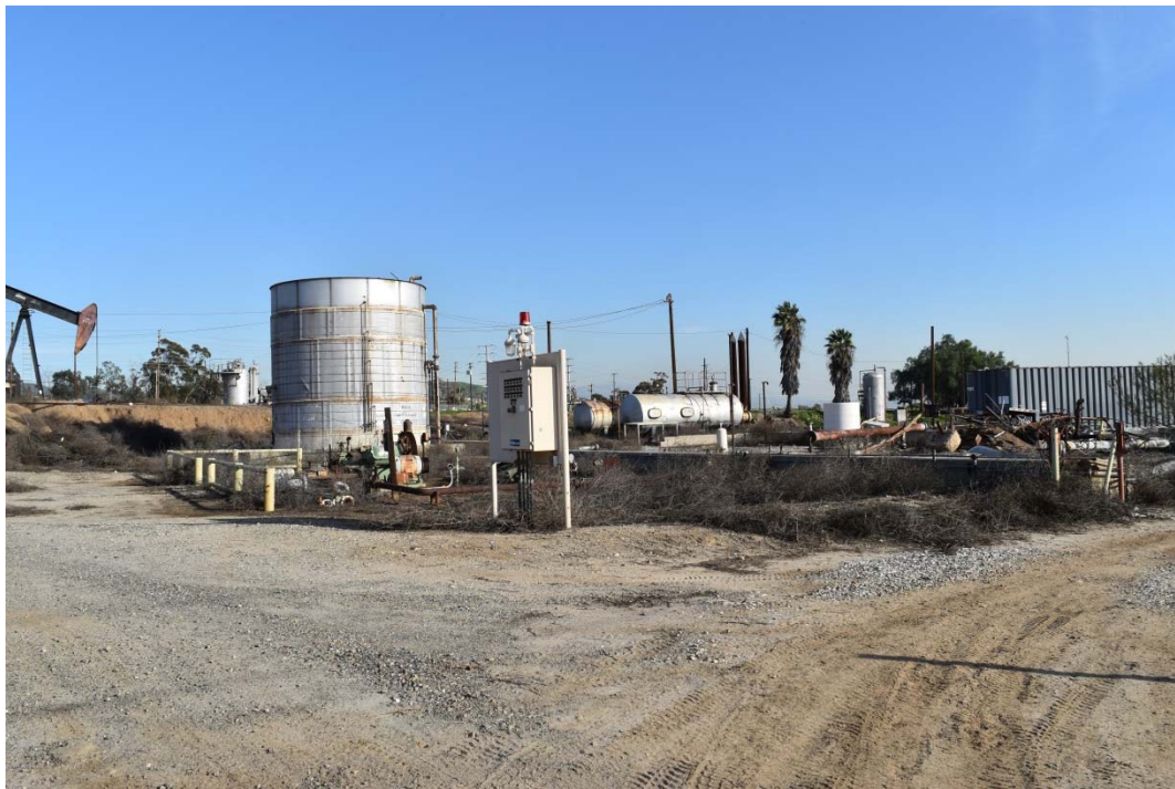
24. Dehydration Unit located in the north central area of the southern portion of the 100-Acre Parcel.
