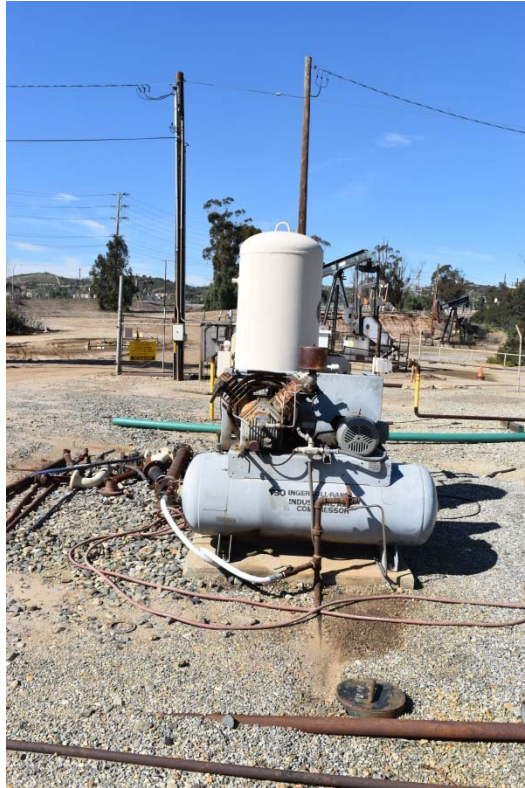
45. Brea Production Unit and Olinda Tank Farm located in the central area of the northern portion of the 165-Acre Parcel.
