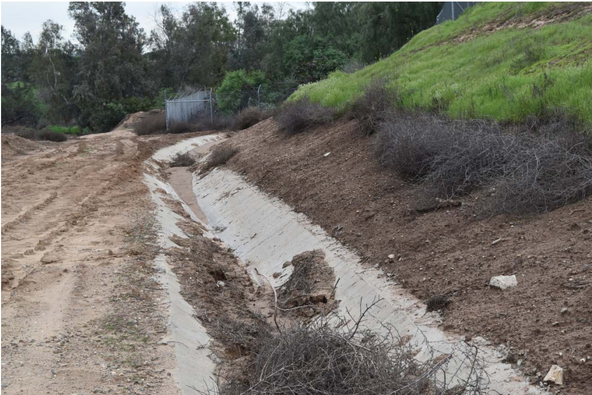
54. Drainage and portion of former sump S20 located in the southern portion of the 165-Acre Parcel.
