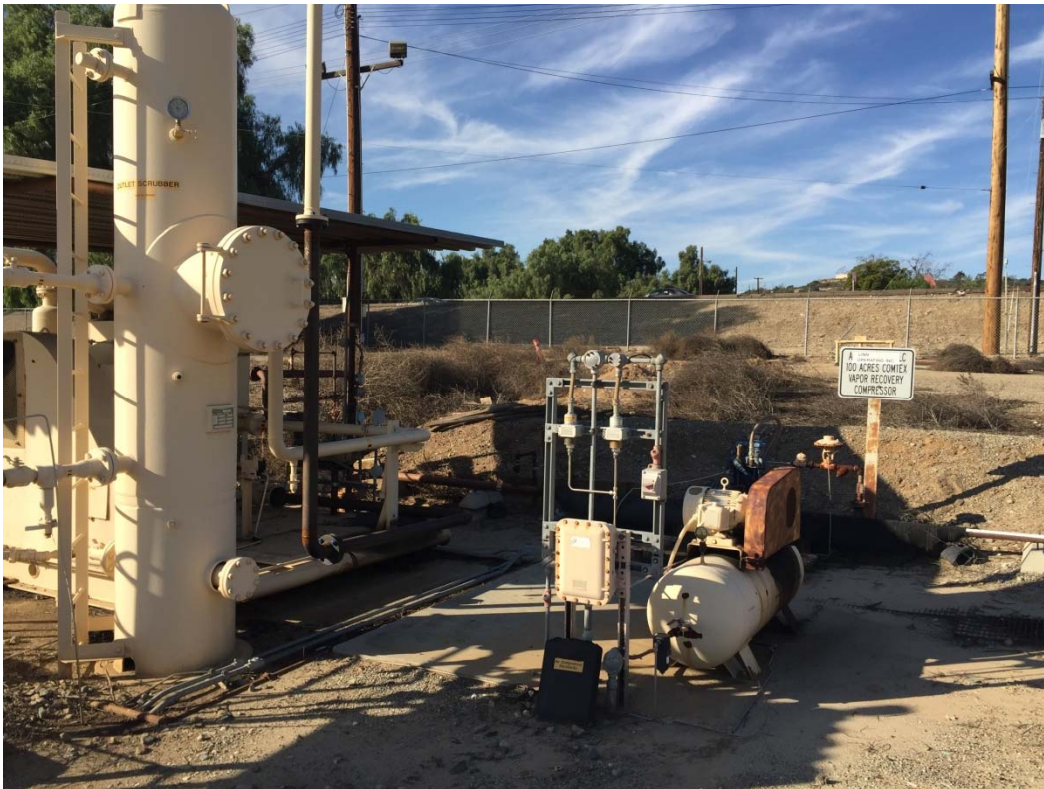
20. Vapor recovery system located in the north central area of the southern portion of the 100-Acre Parcel.
