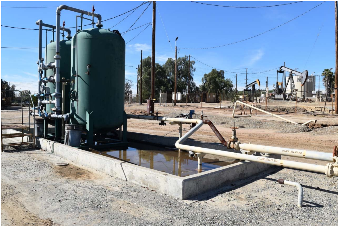
48. Carbon filtration area located in the central area of the northern portion of the 165-Acre Parcel to the south of the Brea Production Unit and Olinda Tank Farm.
