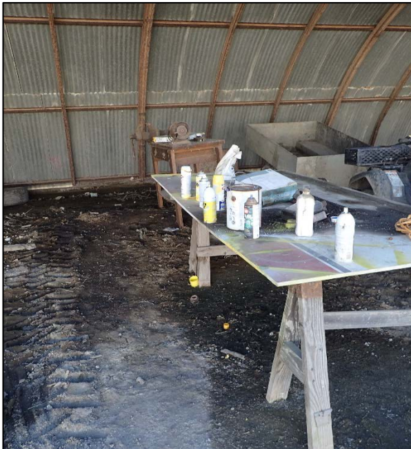
Photograph 15. View of the interior garage (depicted in photograph 21) with significant soil staining and chemical storage.
