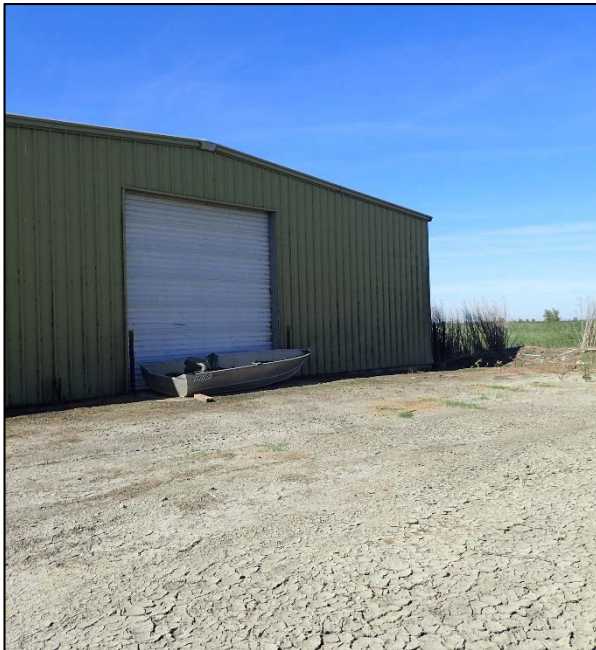
Photograph 23. Warehouse storage building. Concrete foundation, aluminum sided building with roll-up doors (Figure 2d).
