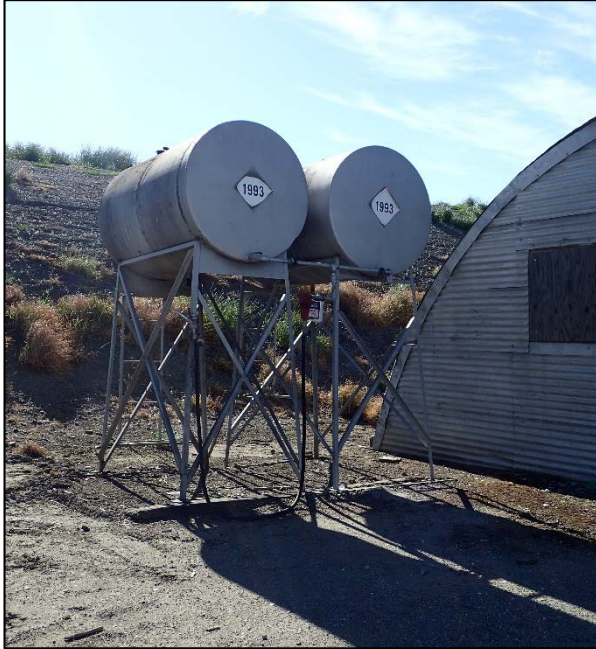
Photograph 13. View of the two active gasoline ASTs located in the developed area near the active warehouse storage area (Figure 2d).
