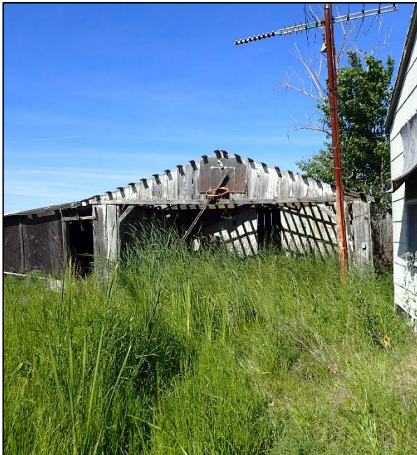
Photograph 47. Dilapidated barn adjacent to residence in Photograph 45 (Figure 2e).
