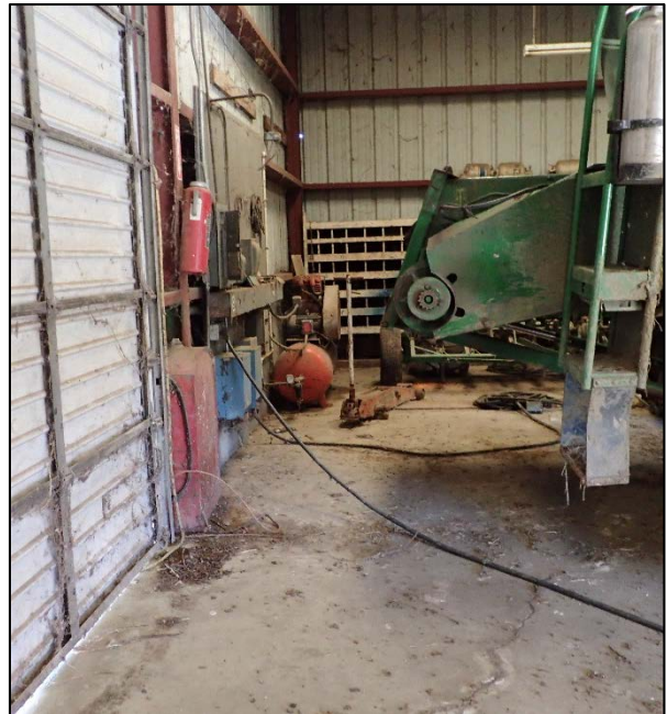
Photograph 28. Warehouse interior, general storage. A small generator (LPG powered) is present, plus fire extinguishers, and corn harvesting equipment (Figure 2d).
