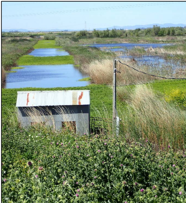
Photograph 67. Abandoned pump house along levee; southern end of Subject Property (Figure 2c).
