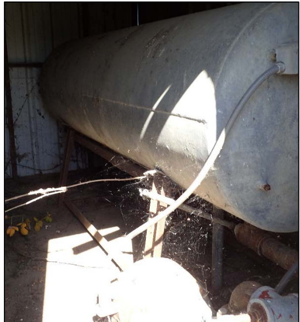
Photograph 32. Abandoned LPG tank, approximately 500 gal. Associated with warehouse. Located outside in an adjacent shed (Figure 2d).
