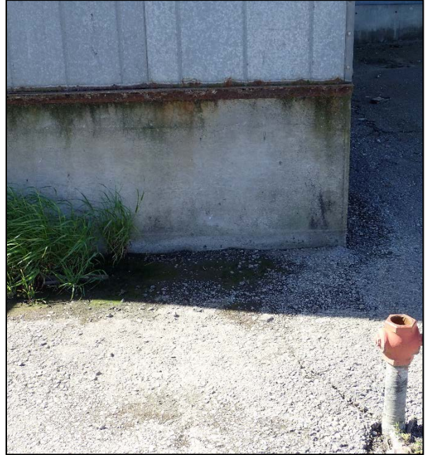
Photograph 38. Pipe of unknown use. Positioning indicates that it may be associated with piping on the building (Figure 2d).
