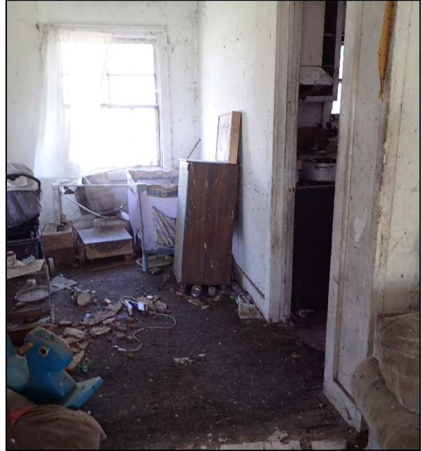
Photograph 46. Abandoned residence interior. Suspect asbestos- and lead-containing materials observed (Figure 2e).
