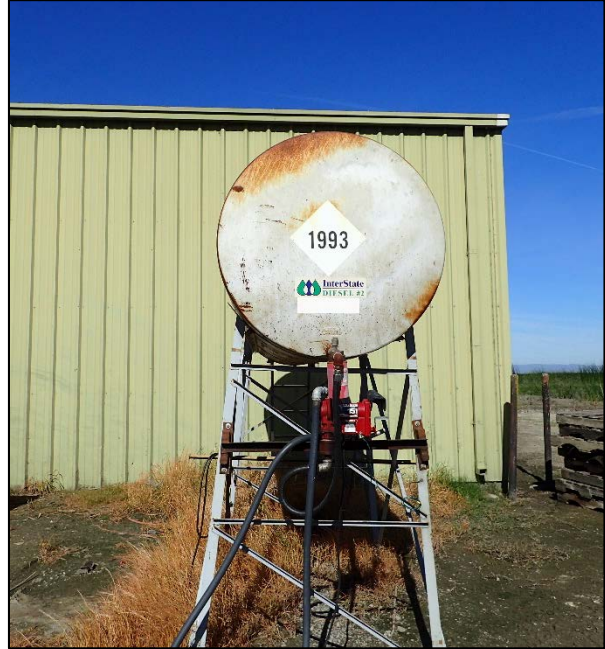
Photograph 34. Diesel fuel AST, approx. 500 gallons, located outside the warehouse. No secondary containment was observed (Figure 2d).
