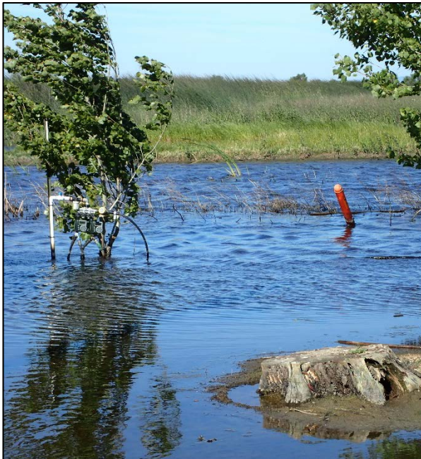
Photograph 11. View of the an irrigation pump located by the caretaker’s residence in the developed portion of the Subject Property (Figure 2d).
